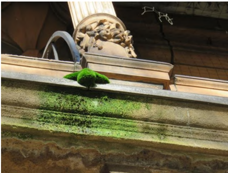
Concentrated algae growth, where water has been directed and contained by obstructions on the cornice. This should be cleaned and any obstruction removed.
