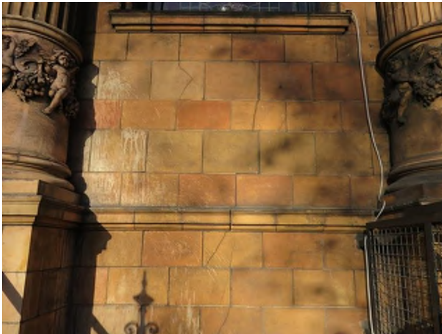
Cracks in the terracotta faience. These could be repaired.
