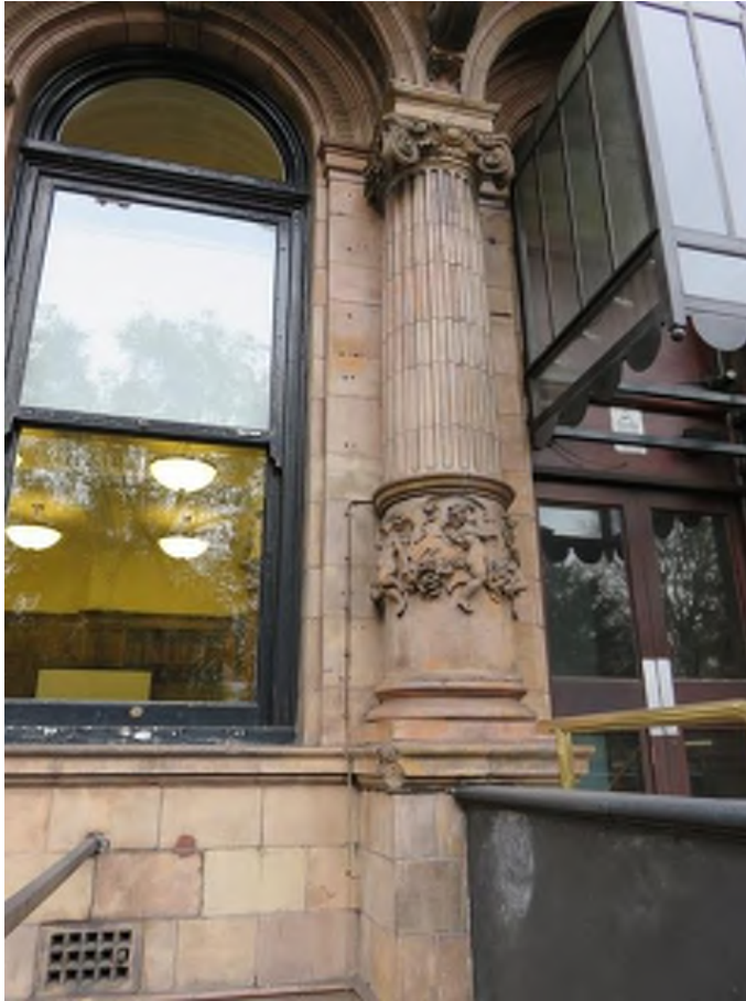
Several hole and nylon plugs in the façade. As they are new an exist they can be repaired.
