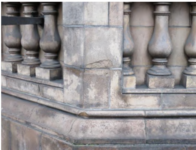
Surface damage. Can be repaired or left as character of the building.
