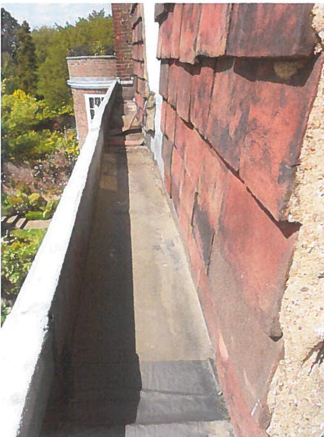
Photo 10 – Rear gutter – patched lead lining
