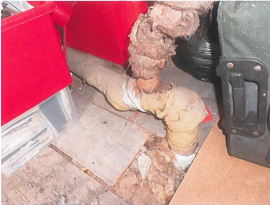
Photo 29 – Asbestos lagging in front roof space
