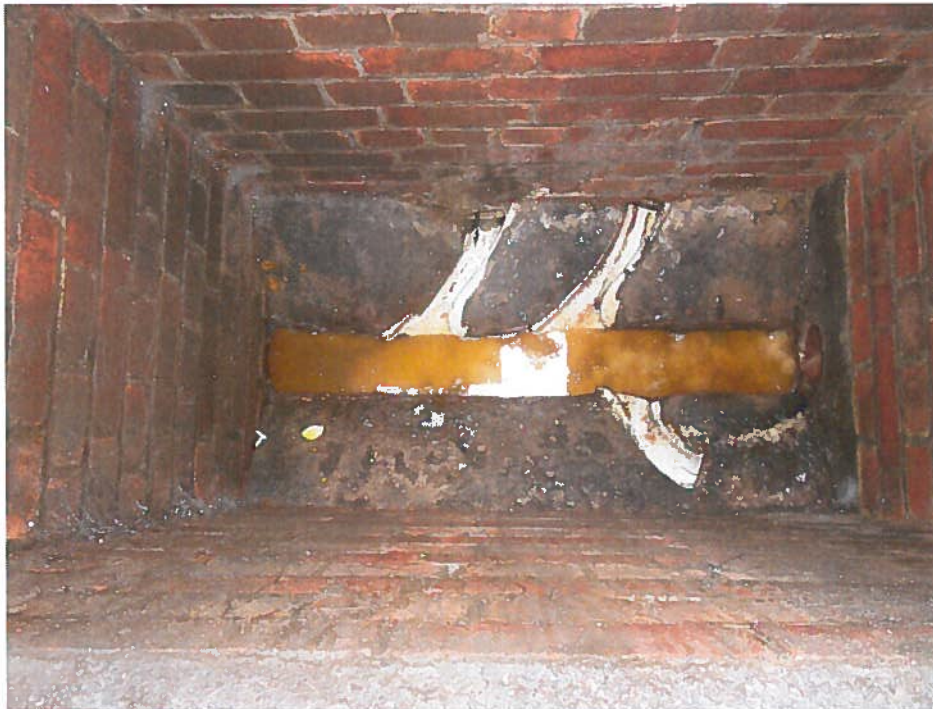
Photo 32 – Blocked channel in manhole
