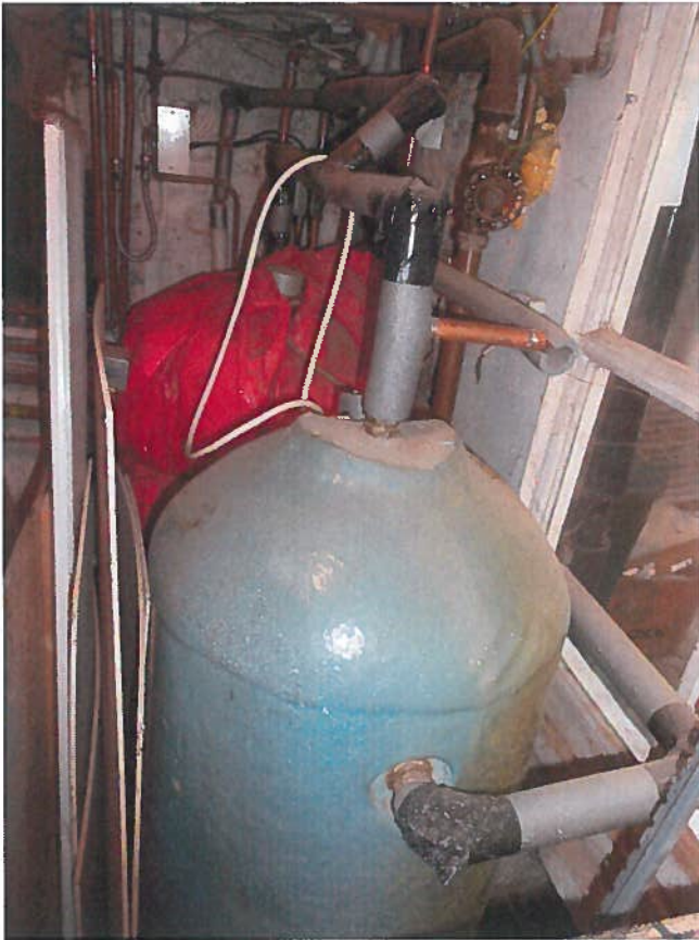
Photo 31 – Hot water cylinders
