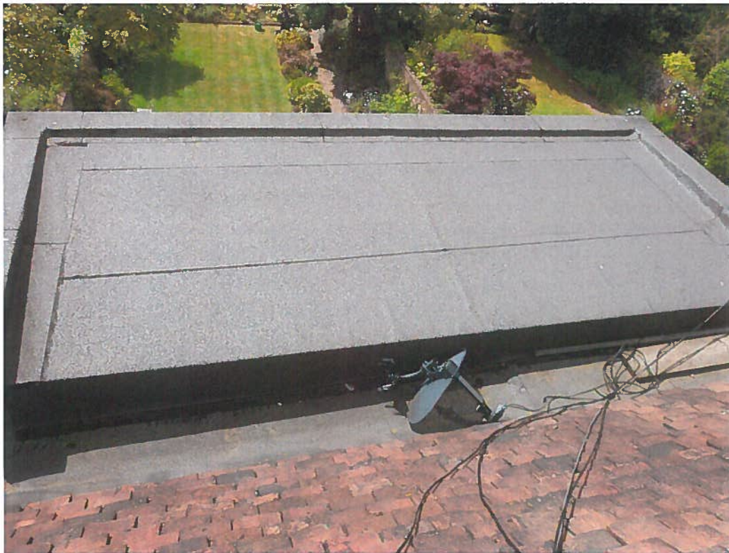
Photo 6 – Flat roof over rear dormer
