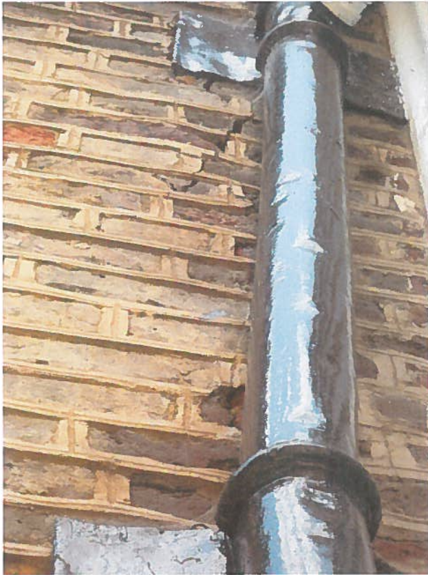
Photo 17 – Close up of repointing on front elevation (old fracture also visible by lead rainwater pipe)
