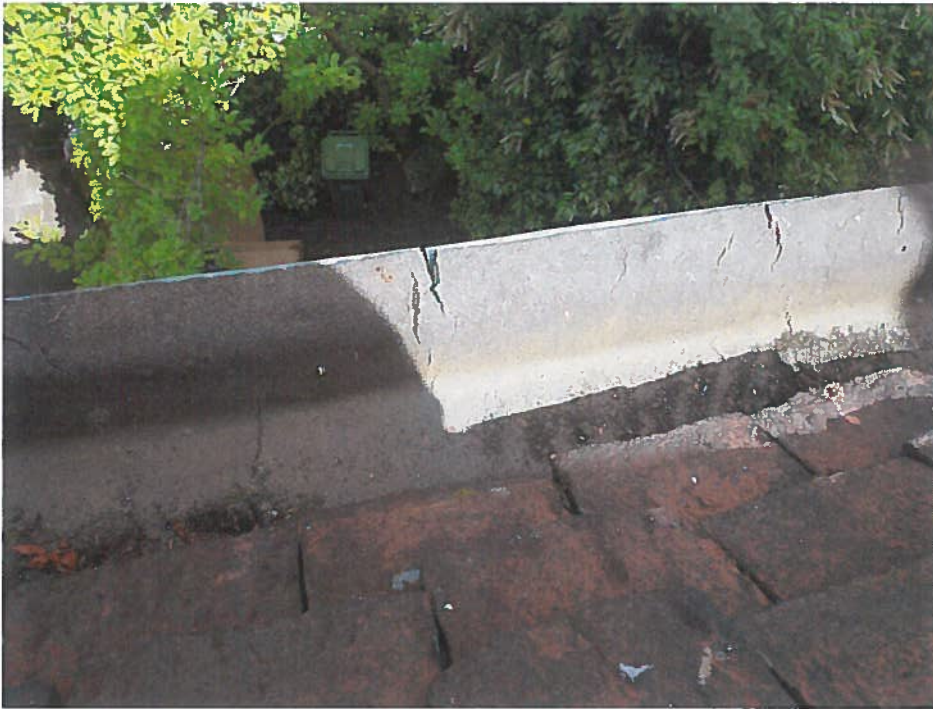
Photo 9 – Front gutter – splits in asphalt lining
