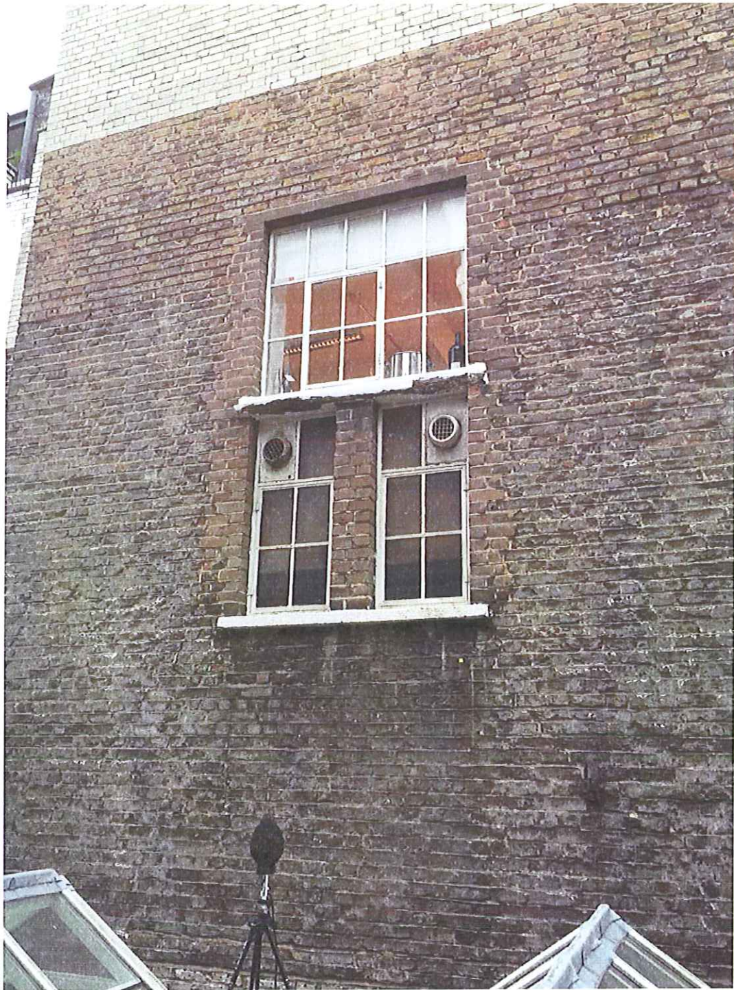
Photo E – View of Nearest Window to Rear of Site (Office Window)
