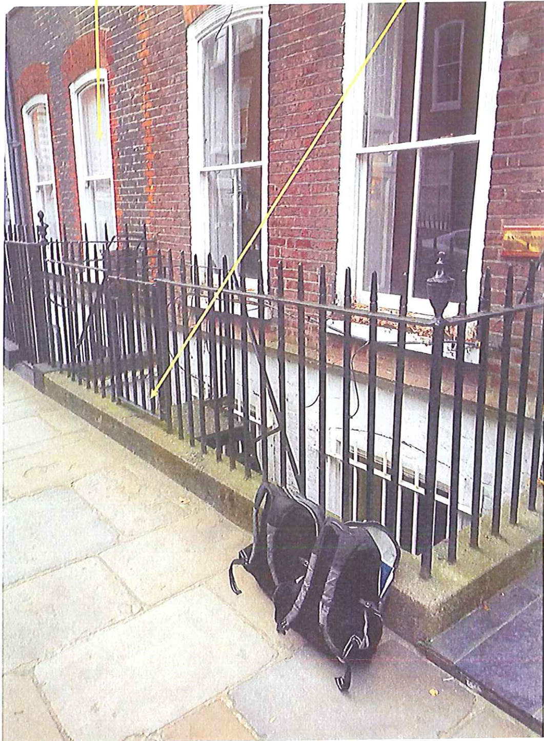
Photo D – Basement Area at Front of Building with Plant Vault Under Pavement
