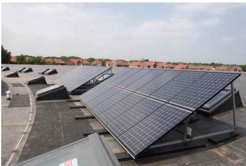
Figure 1: Roof mounted photovoltaic panels
