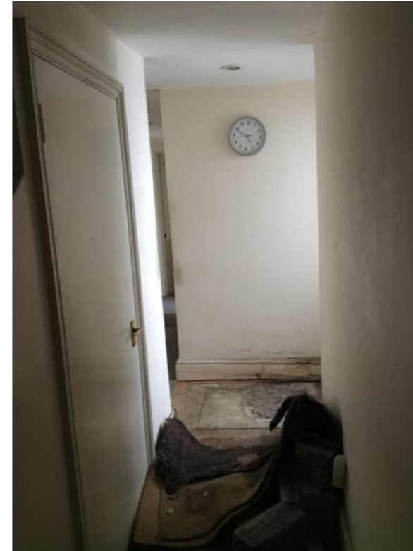
Fig 3: Damp to lower ground floor rear corridor
