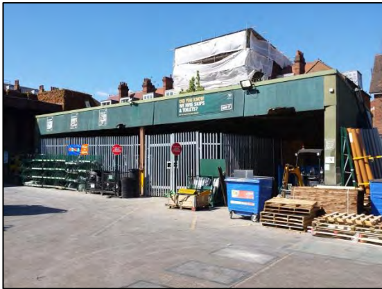
Figure 32: Metal framed and clad structure used as a hired plant store. Viewing ~ NW
