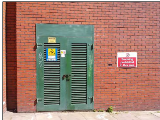
Figure 4: Electrical Substation located in the north western corner of the site, within the 'northern' Council office buildings. Viewing ~ E
