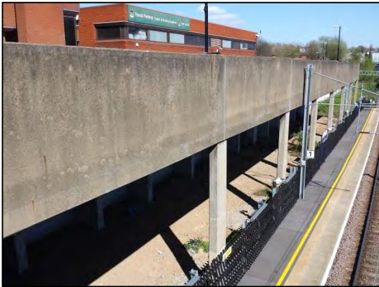
Figure 9: Concrete columns and land underneath the floating deck adjacent to Platform 1. Viewing ~ NE
