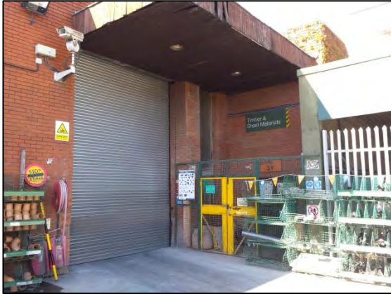
Figure 30: Red brick extension to the warehouse with adjacent metal structure. Viewing ~ NW
