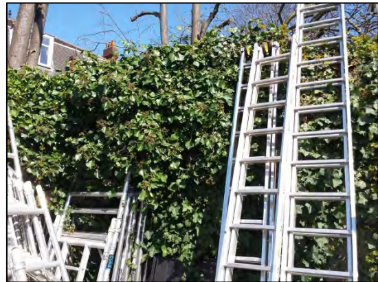
Figure 14: Significant visible growth of ivy and buddleia on the northern and eastern boundary walls in the north eastern corner of the site. Viewing ~ NE
