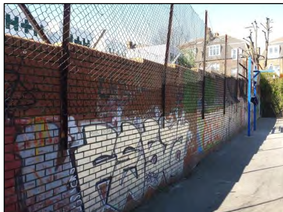
Figure 12: Red brick wall which formed the eastern site boundary, viewed from the off-site sports court. Viewing ~ NW
