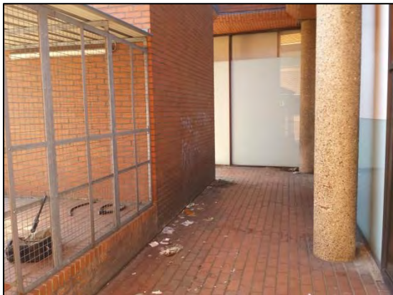
Figure 5: Walkway around the metal storage cage adjacent to the single storey section. Viewing ~ W
