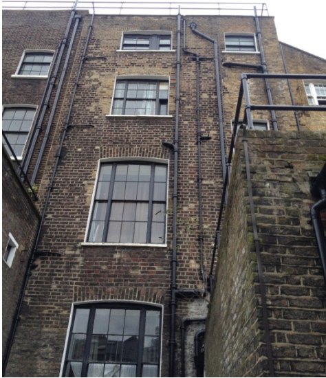
Figure 2: No. 66 Guilford Street, rear elevation showing historic windows and rear closet wing.
