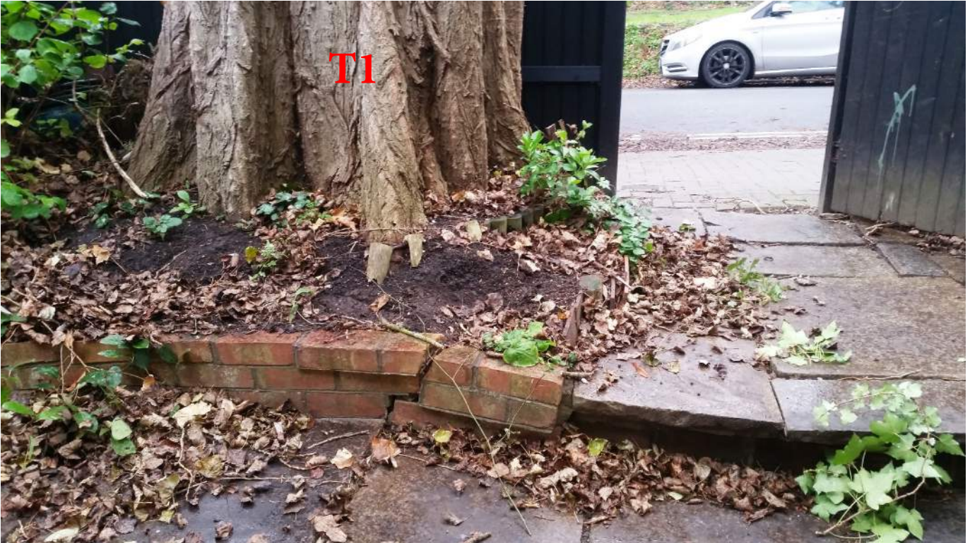
Base of tree T1 showing butress roots and existing entrance with level change step
