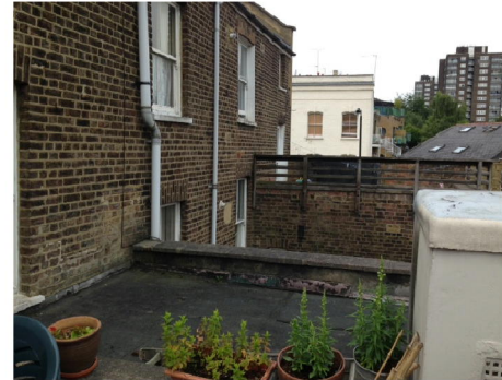
PHOTOGRAPH 2 - Existing flat roof of 6 Mansfield Road in the foreground with an existing roof terrace with timber guard railing at 4 Mansfield Road beyond.
