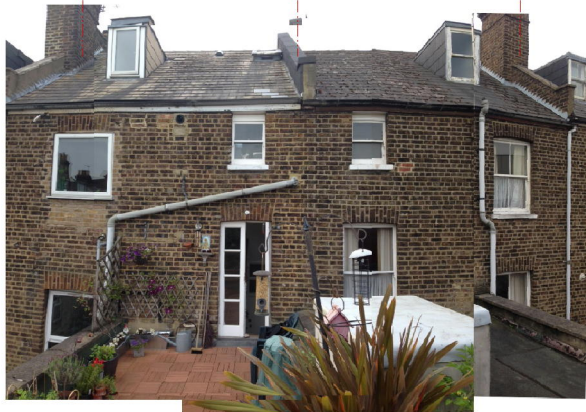
PHOTOGRAPH 1 - Composite panorama photograph showing the existing unguarded roof terrace to the rear of 8 Mansfield Road and the adjoining flat roof to 6 Mansfield Road.
