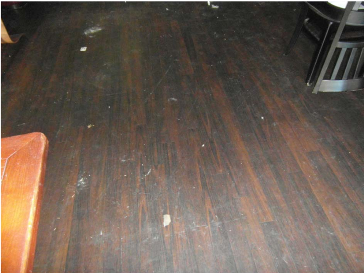
Ground Floor Non-Original Flooring
