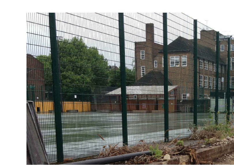
Existing 5m high ball fence to be retained and made good where removed.
