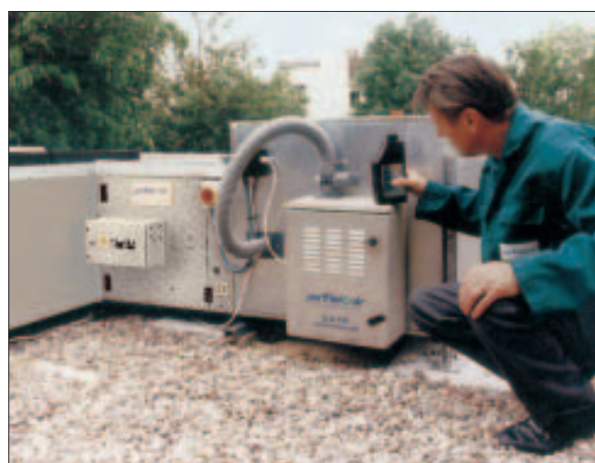
The O.N.100 in situ on a flat roof installation with the ESP 3000 E Pre-filtration unit.
