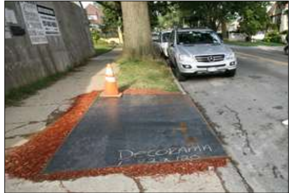
Photo 14: Steel plates can be an effective way of temporarily reinforcing weak surfacing over a construction access during the development activity.
