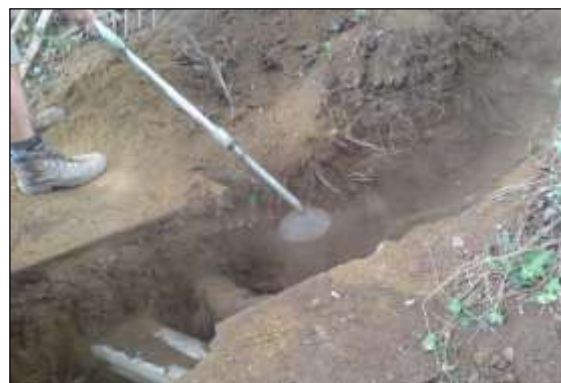
Photo 16: Air spades are very effective at exposing roots and services with minimal damage.
