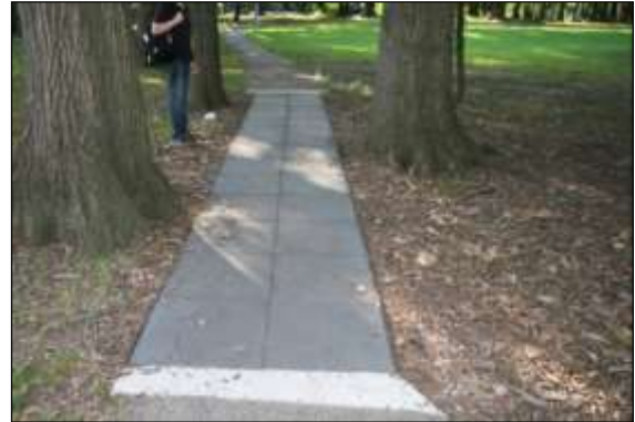
Photo 33: Where surfacing is needed close to rapidly growing buttress roots, a light metal frame with rubberised surfacing will allow the path to distort without cracking as the roots grow.
