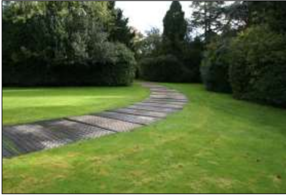
Photo 19: Ground protection must be used where repeated foot or vehicle traffic could cause compaction in sensitive RPAs. It can be as simple as plywood for pedestrians, but must be more robust for vehicles.
