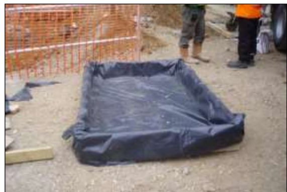
Photo 47: Soil bunding or a supporting framework covered in heavy-duty plastic sheeting is essential where there is a risk of spillages contaminating RPAs. This specifically applies to cement mixing areas and vehicle washing facilities.
