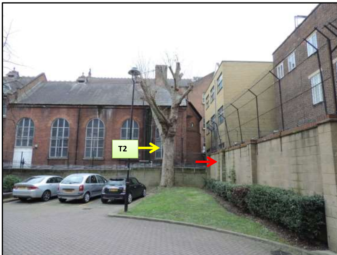
Image 2: The existing boundary wall (red arrow) is likely to be providing a deep barrier for root growth
