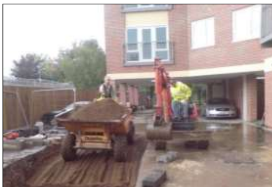
Photo 53: Structural tree soil retains sufficient structure for tree roots to grow, even when compacted.
