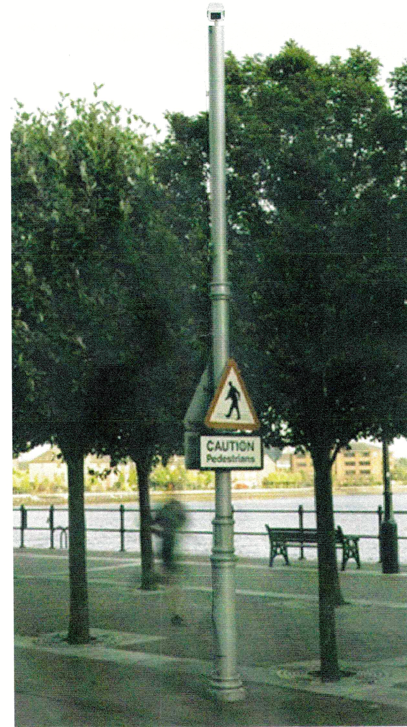
TYPICAL EXAMPLE OF A SIMILAR CAMERA COLUMN INSTALLATION
