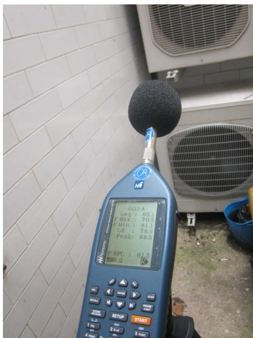
Figure 6 –Measurement Position P2 used for determining source noise levels ( L_{Aeq} ) of existing condensers
