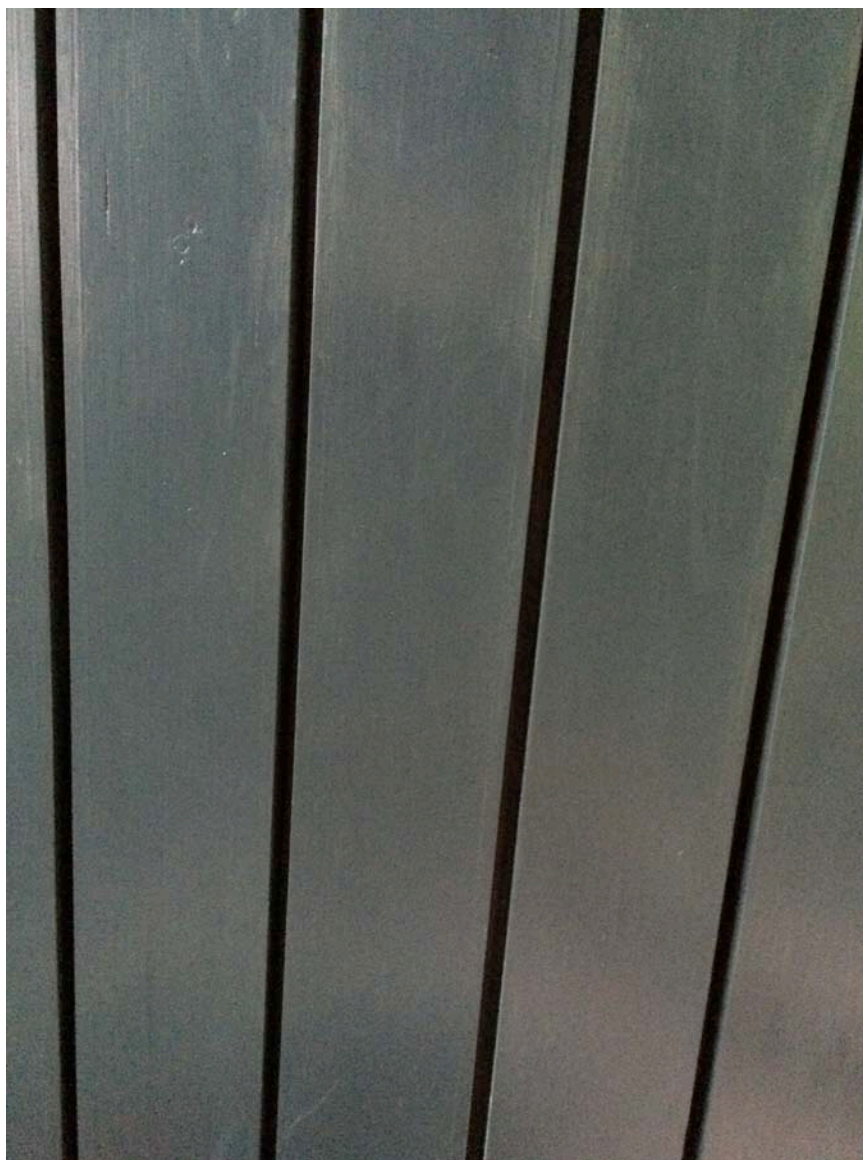
Close up of painted timber boarding RAL 7016 Anthracite grey with 10mm shadow gaps between boards.
