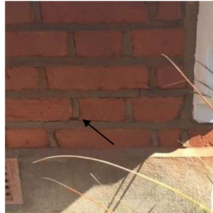
Diagonal stepped cracking to ground floor bay.
