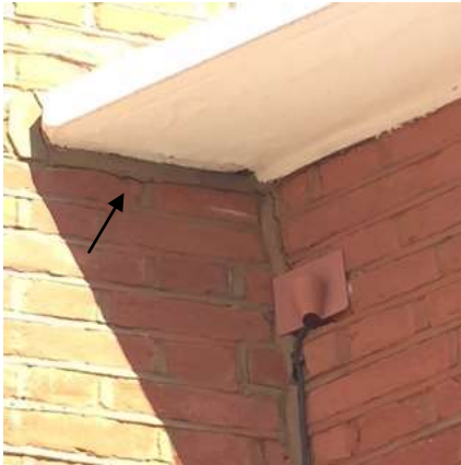
Separation to abutment of bay.
