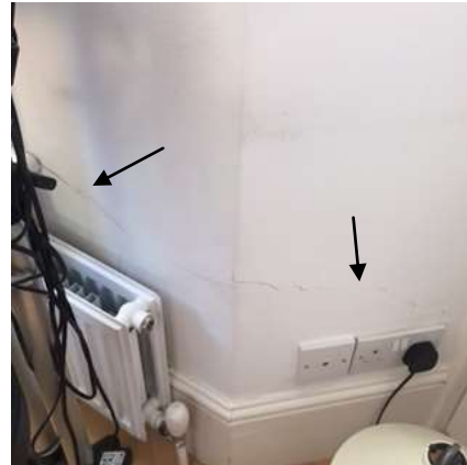
Diagonal cracking to ground floor bay.
