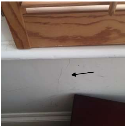
Diagonal cracking below bay window to first floor flat.
