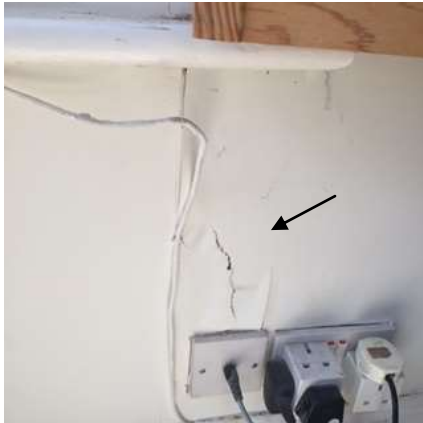
Diagonal cracking to first floor bay.
