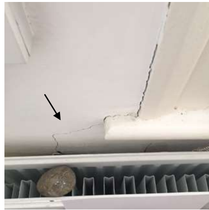
Diagonal cracking below bay window to ground floor flat.
