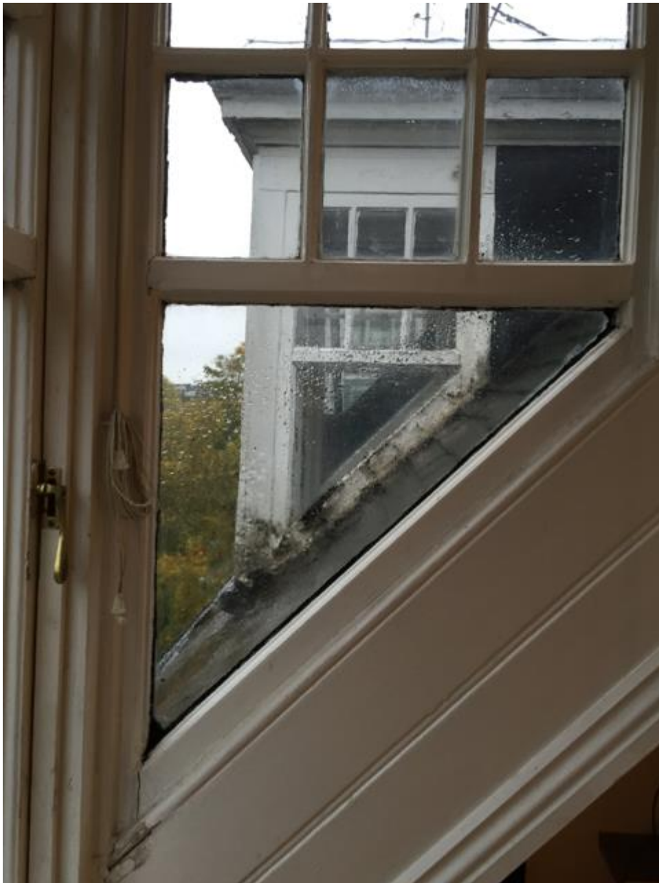
View from the living room, rotten wood visible
