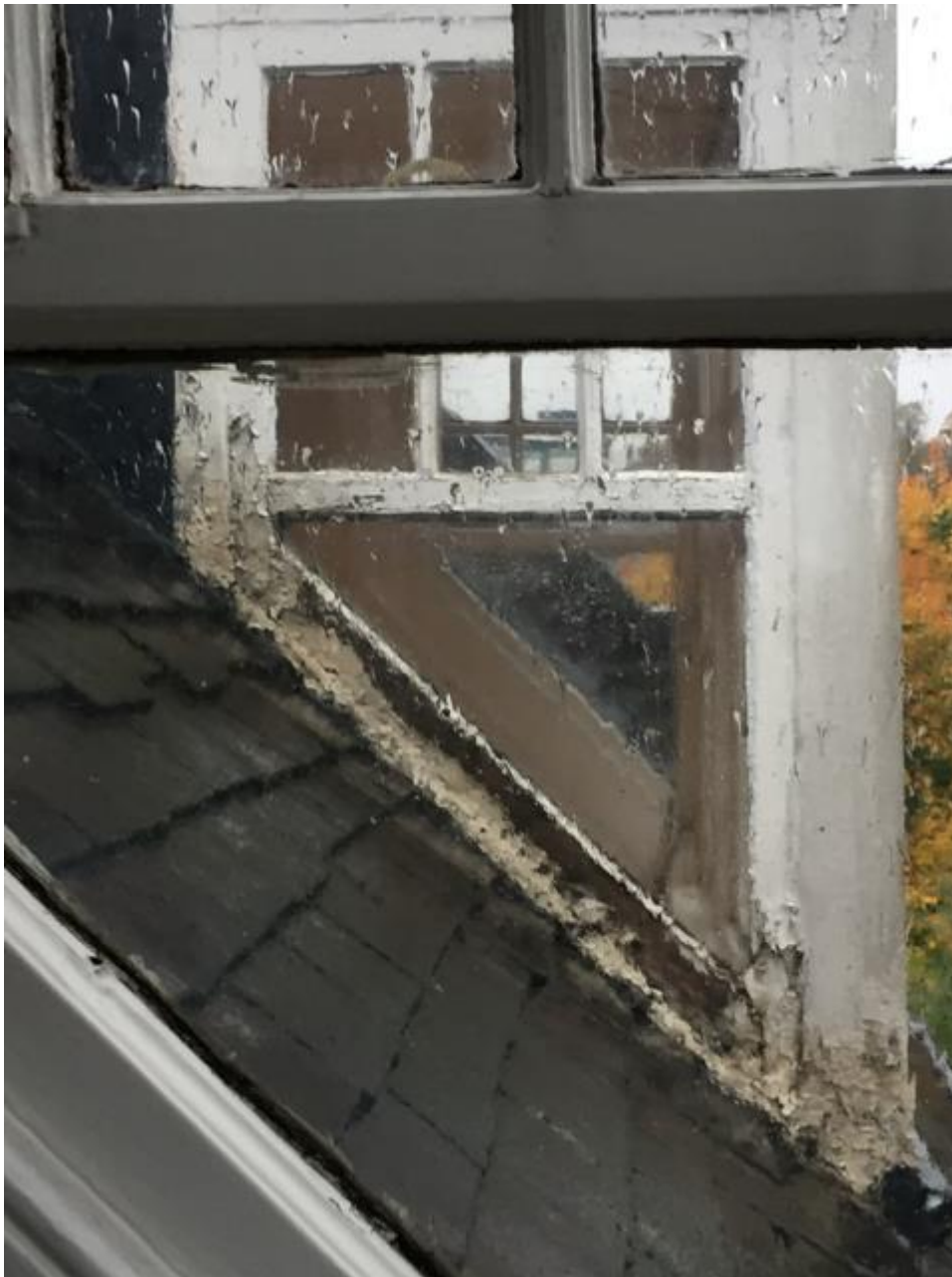
View from the bedroom, rotten wood
