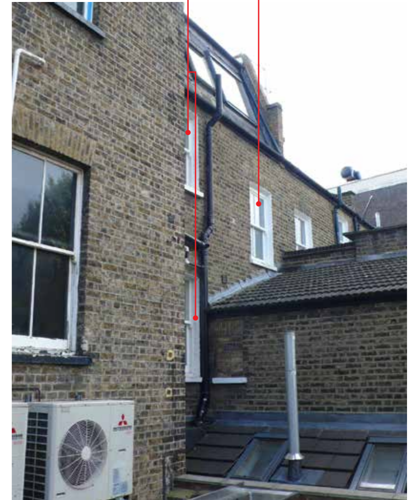
Photograph showing rear windows of 1 Highcroft in relation to the site for the flats.
