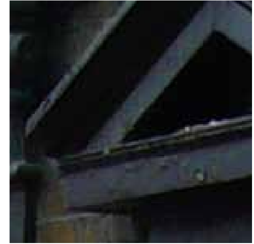
Brown painted fascia
