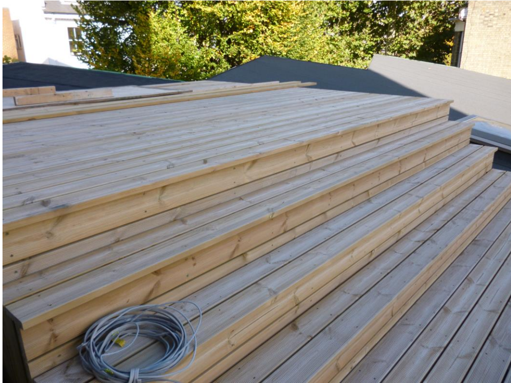
View of steps and raised area of the roof terrace taken next to the access door
