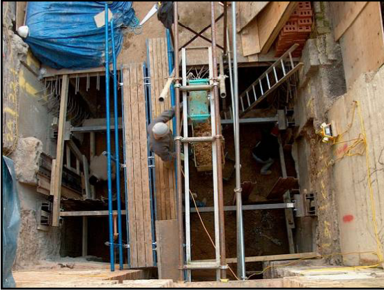
Smith Street, SW3: Two storey basement under existing house on very tightly constrained site with neighbouring 6 storey buildings.
