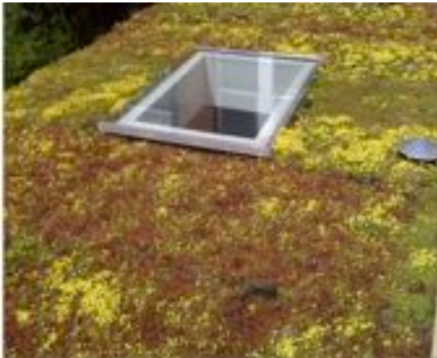
Image of sedum green roof as proposed for the rear extension roof top
