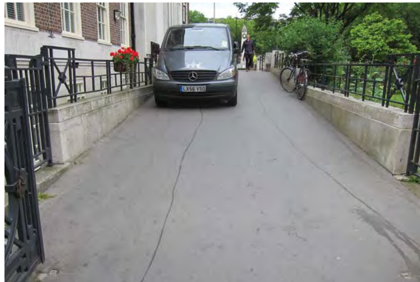
Ramped access (approx 1:15) is non DDA compliant and misses an opportunity to create a welcoming approach to the main entrance.
