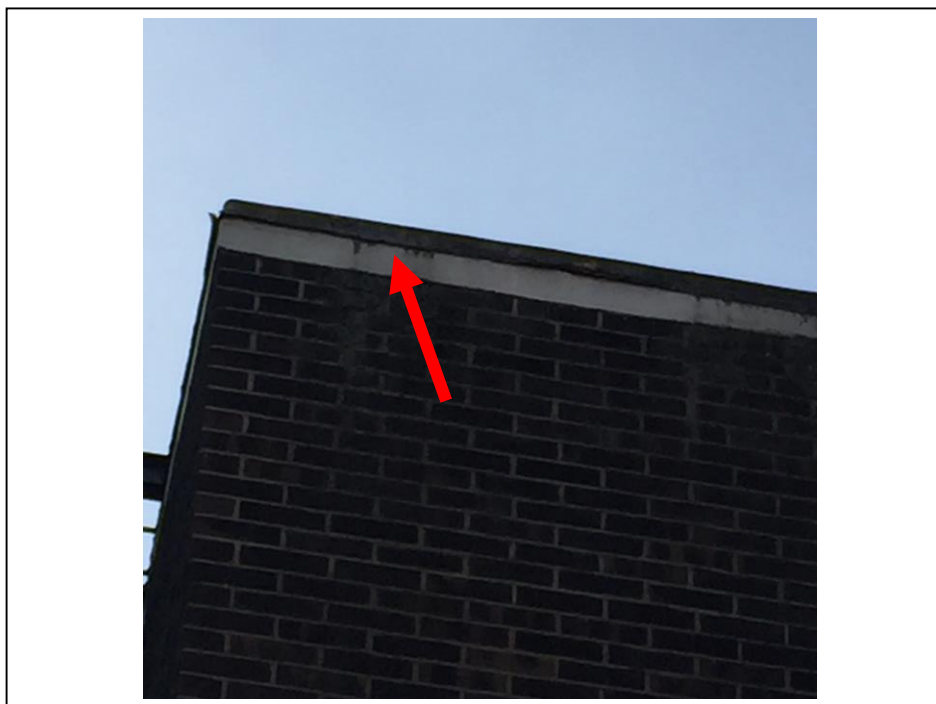
Photograph 10 – Lifted Lead Flashing: Covered Stairwell (Devonshire Court)
