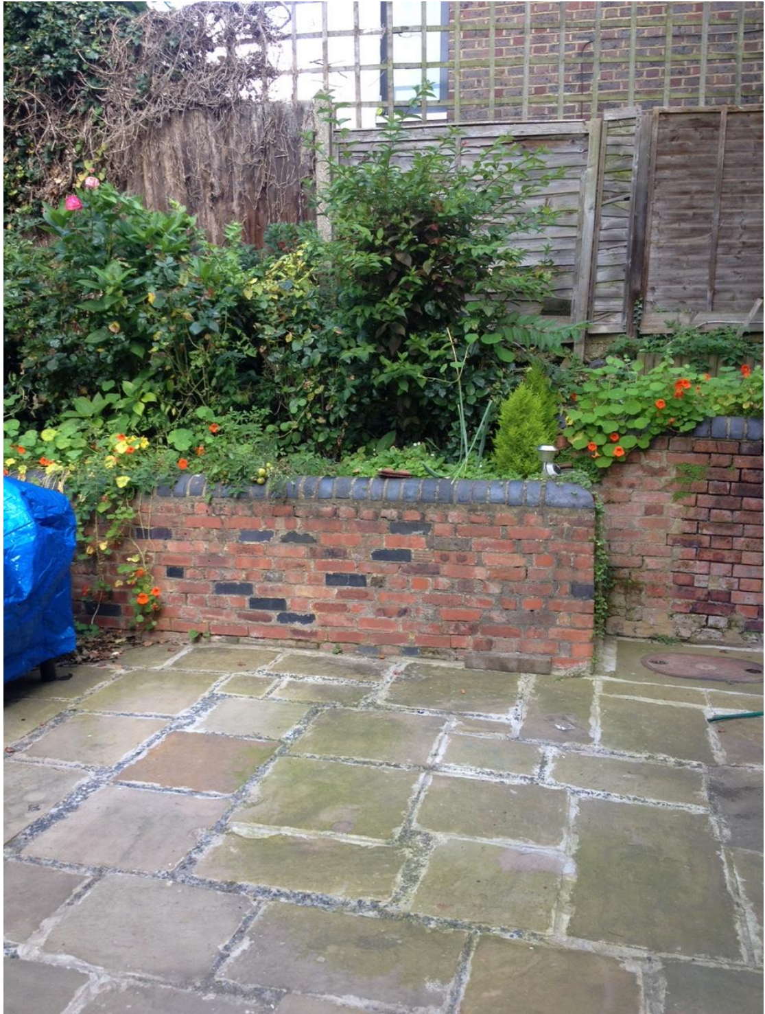
Photo 3- Retaining wall to be pushed back to match line of wall section on right hand side
