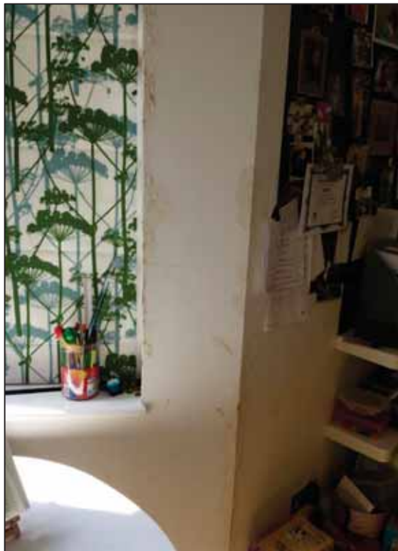
Figure 10: Wall damage to wall in breakfast area
