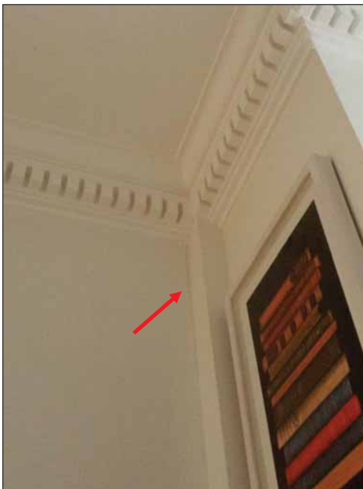
Figure 12: Vertical crack in the wall - dining area
