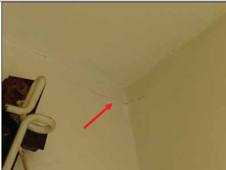
Figure 11: Example of minor cracking
