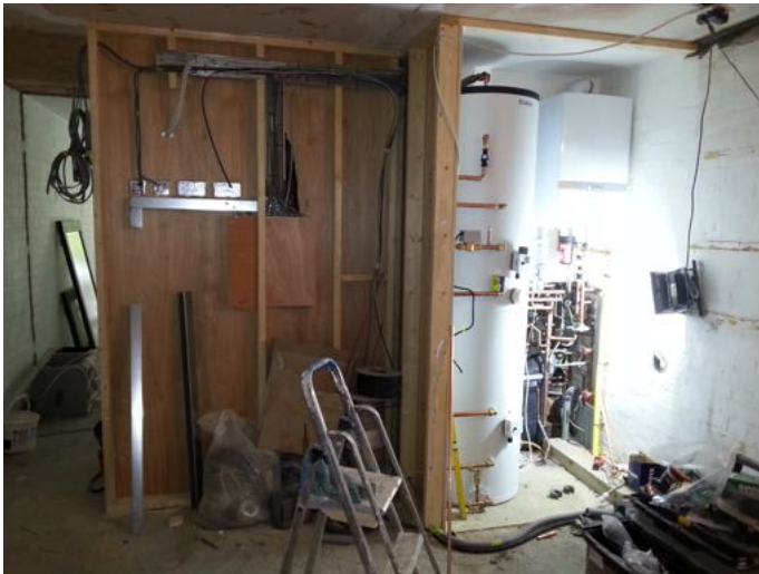
below stairs plant area
