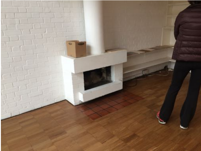
living room concrete fireplace with asbestos flue
