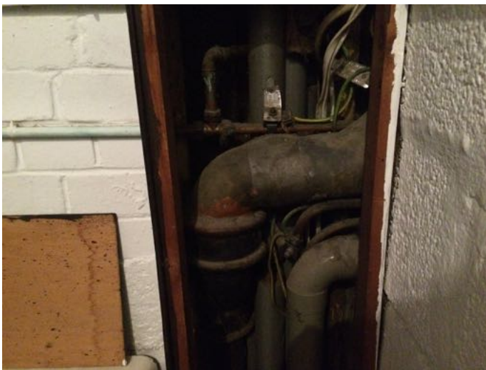
inside of service riser in stairs
