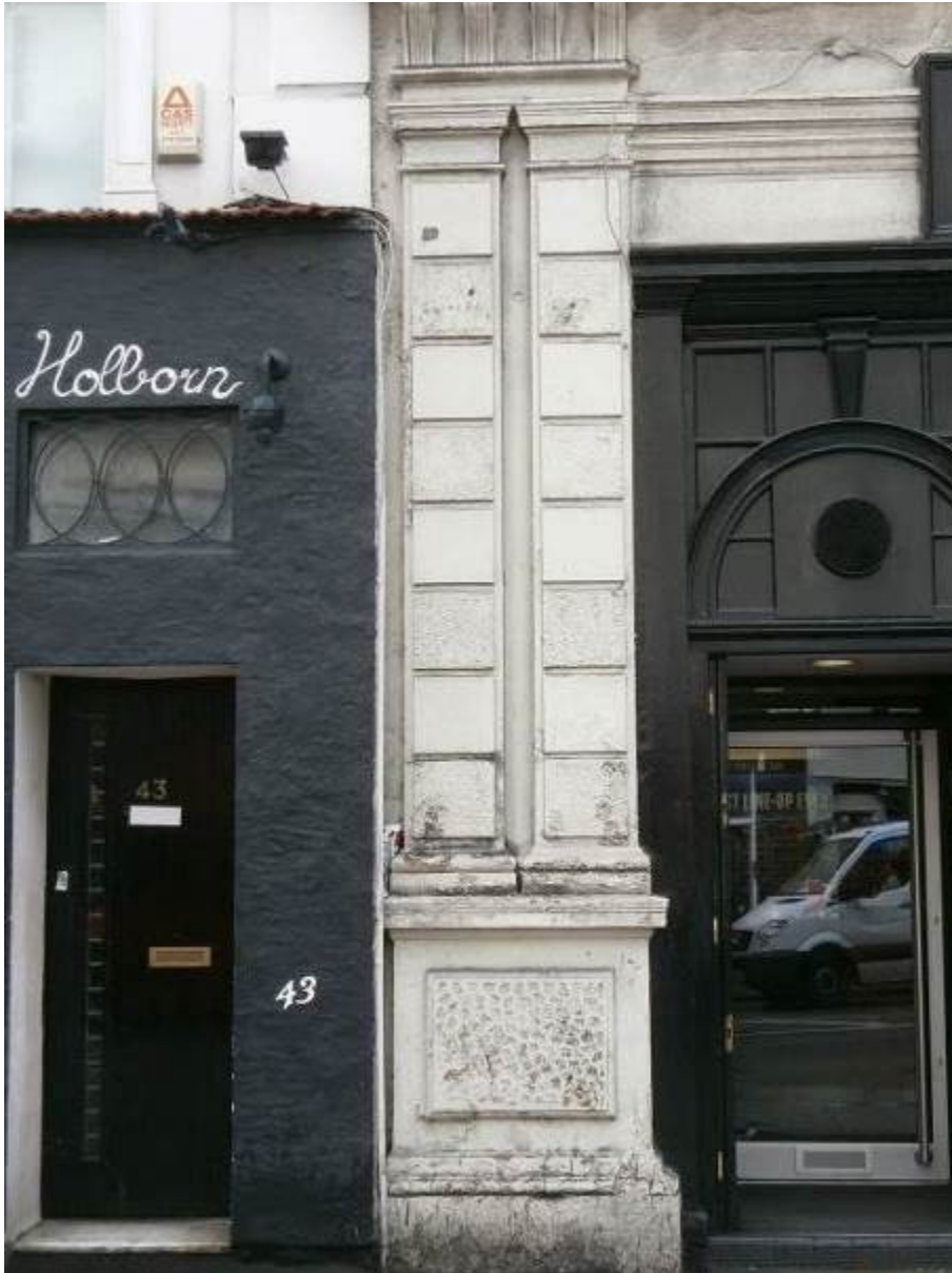
Front Elevation – Ground Floor – flaking decoration and sub-fluorescence to plinth. Paint-obscured vermiculated render panels.
