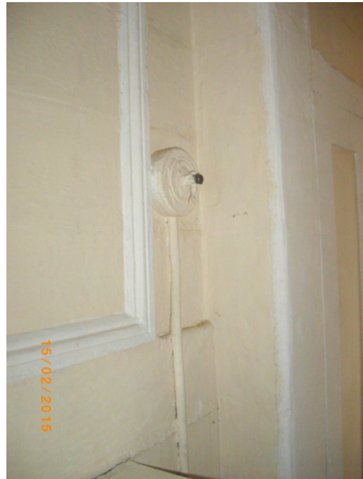
Gas supply for gas lighting, 1 st Flr.
