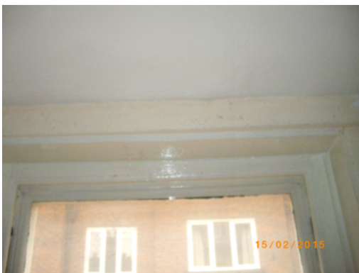
Window surround 2 nd Flr Front Room
