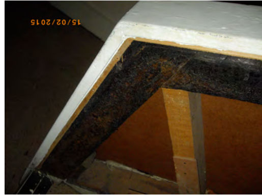
Handrail charred badly
