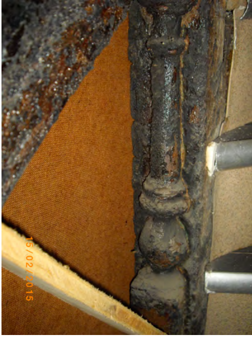
Damage to Staircase, covered with hardboard.
