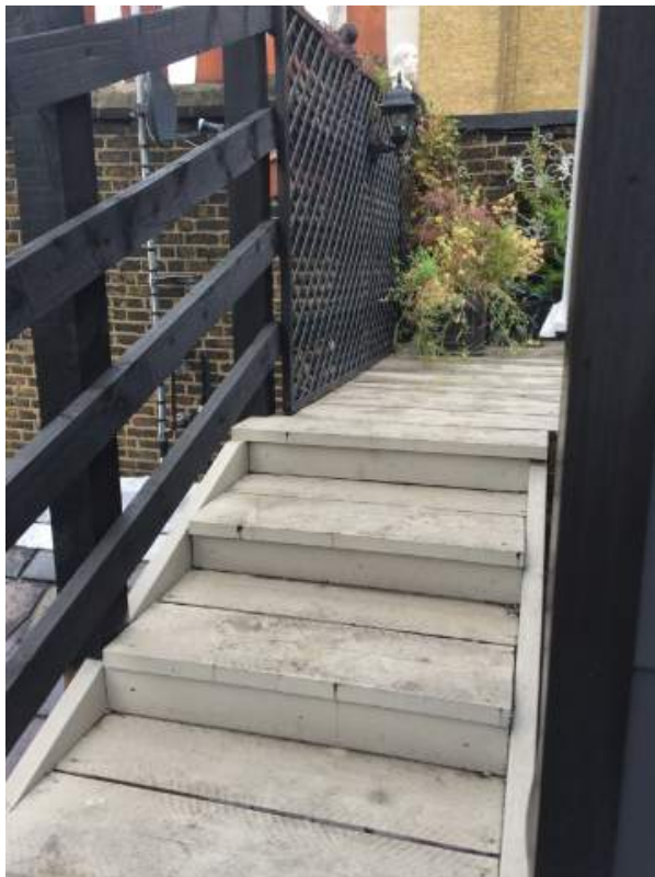
Photograph showing staircase to roof terrace with decking and balustrading (taken from bottom of stairs to the roof terrace looking East)
