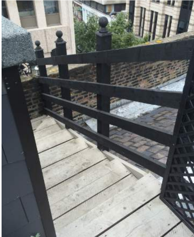
Photograph showing staircase and balustrading (taken from top of stairs to the roof terrace looking West)
