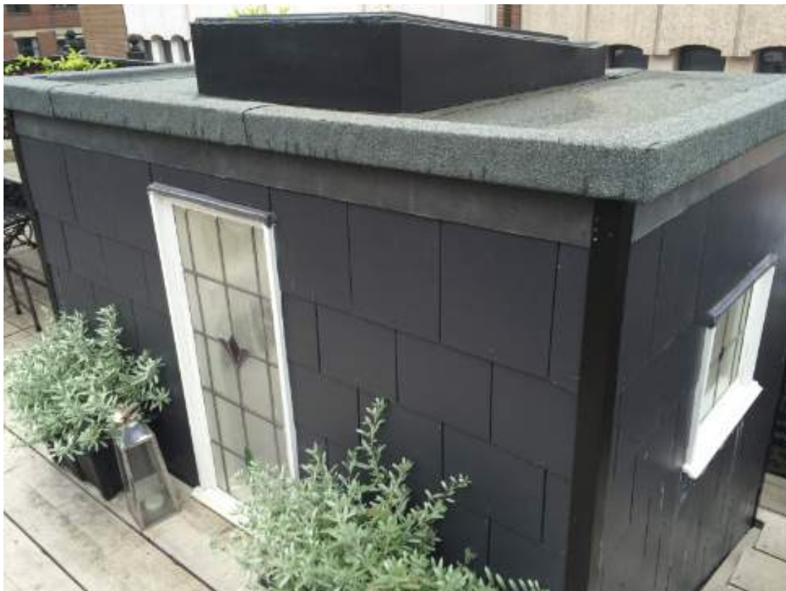
Photograph showing dormer entrance to roof terrace with decking (taken from top of stairs to the roof terrace looking West)
