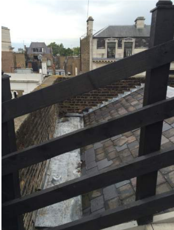
Photograph showing balustrading and existing roof (taken from bottom of stairs to the roof terrace looking North)
