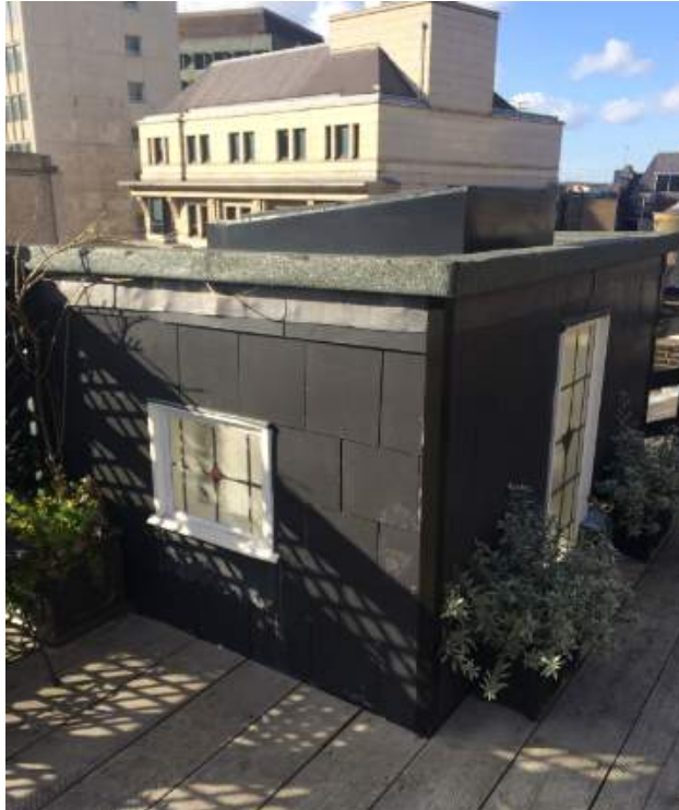
Photograph showing dormer entrance to roof terrace with decking (taken from middle of roof terrace looking North West)
