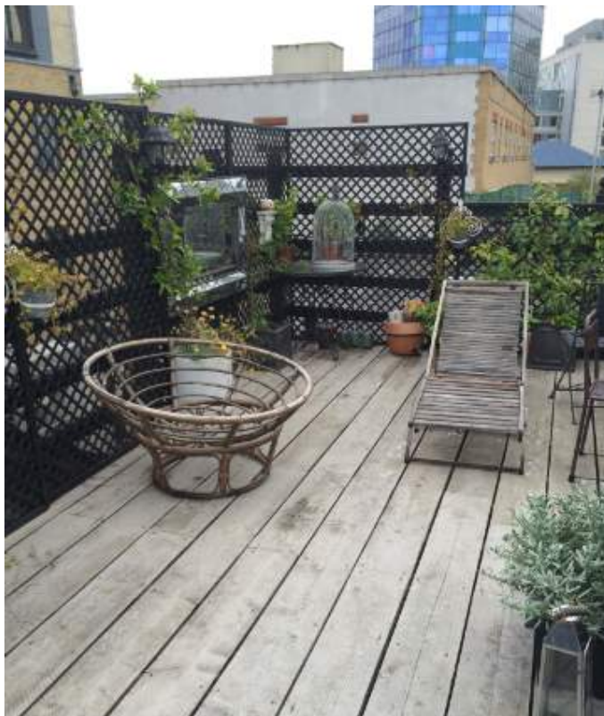
Photograph showing roof terrace with decking and balustrading (taken from top of the staircase looking South East)
