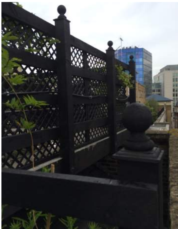
Photograph showing balustrading and setback from parapet on Newton Street (taken from entrance to roof terrace looking South)
