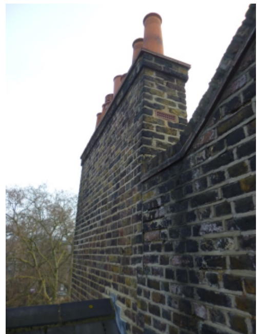
4. Stack clearly leaning away from the roof of no 21.
