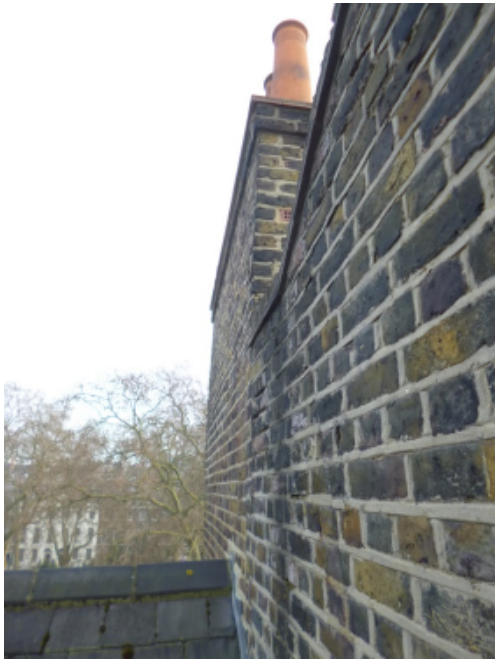
5. Upper section of stack clearly leaning.
