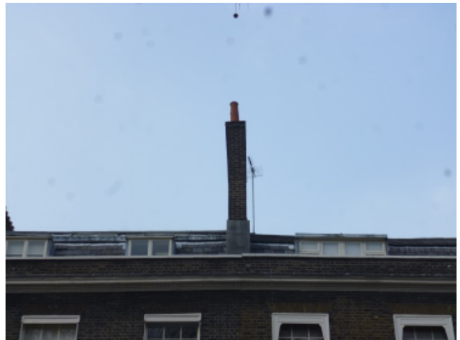
2. Party wall stack on left hand side (no 21/22) clearly leaning.
