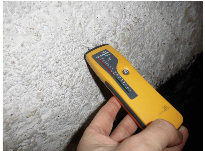
Photograph 4 - High damp readings taken to wall on line of hatch
