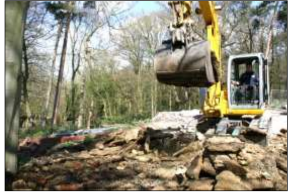
Photo 20: Machines with a long reach can be used to lift out heavy surfacing and structures as long as the machine sits outside the RPA and the exposed surface is protected before there is any further access.
