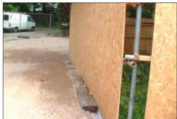
Photo 27: Although this is only a temporary surface, railway sleepers pinned into the ground can be used to retain the edges of new surfacing.
