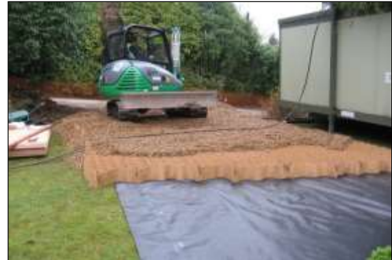
Photo 25: The stone-filled cells spread the load of traffic and the geotextile membrane on the ground prevents migration of the stone into the soil profile.
