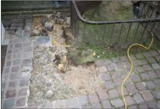
Photo 21: Careful lifting of cemented-in sets round this tree allowed them to be re-laid on a permeable sand base, improving the water input into the soil around the trunk.
