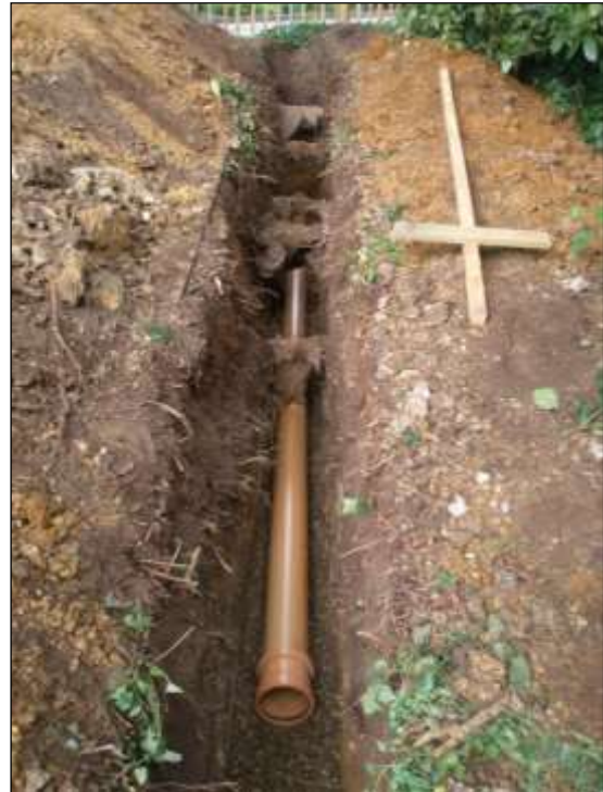
Photo 45: Continuous trenches dug by hand so that important roots can be retained (with the service ducting threaded beneath) is an effective means of minimising damage (note the ground protection boards with soil piled on top on the left).
