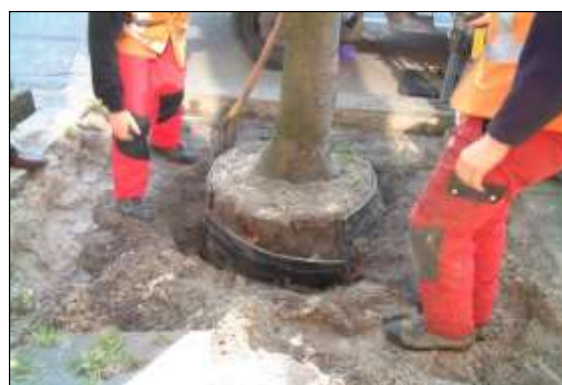
Photo 58: This excavated tree shows the root deflectors that were installed when it was planted seven years previously. The product has deflected roots downwards and prevented damage to the adjacent surfacing. Note that this is a permeable sandy soil and the roots were able to grow beneath the bottom of the deflectors.
