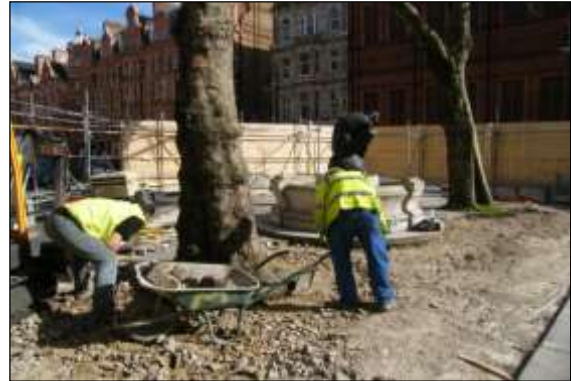
Photo 22: These trees had impermeable surfacing right up to their trunks, which had to be removed by hand before installing new structures.
