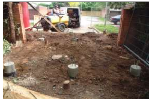
Photo 41: Piles can also be used to support bridges across sensitive RPAs, but the temporary ground protection has to be removed before the main structure is either imported in or cast on site.
