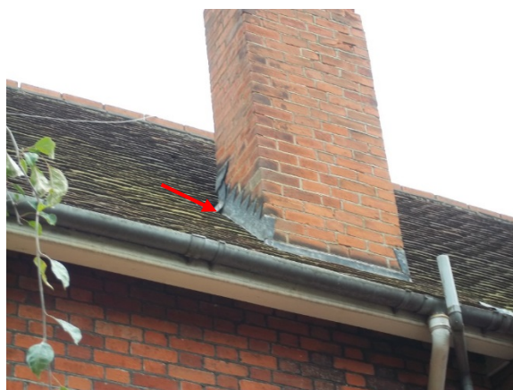
Plate 3.11: Lifted lead flashing
