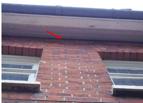
Plate 3.10: Gap at soffit box
