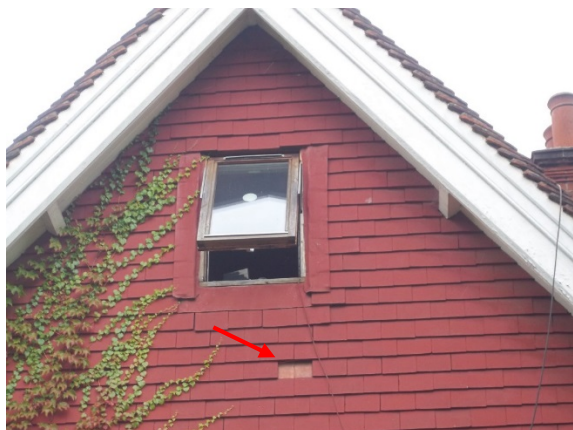
Plate 3.8: Missing hanging tile
