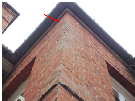
Plate 3.9: Lifted wooden fascia
