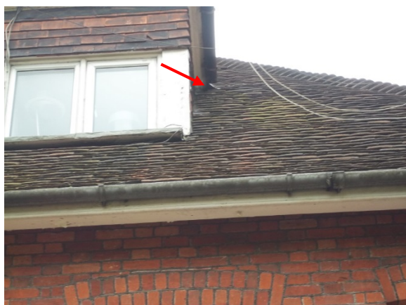
Plate 3.12: Lifted lead flashing
