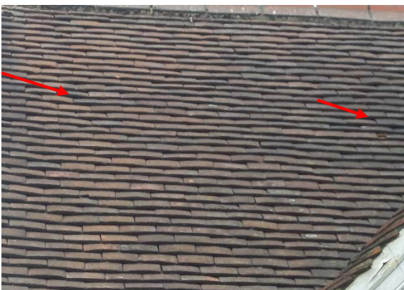
Plate 3.6: Gaps under roof tiles
