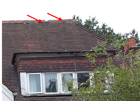
Plate 3.7: Gaps under ridge tiles
