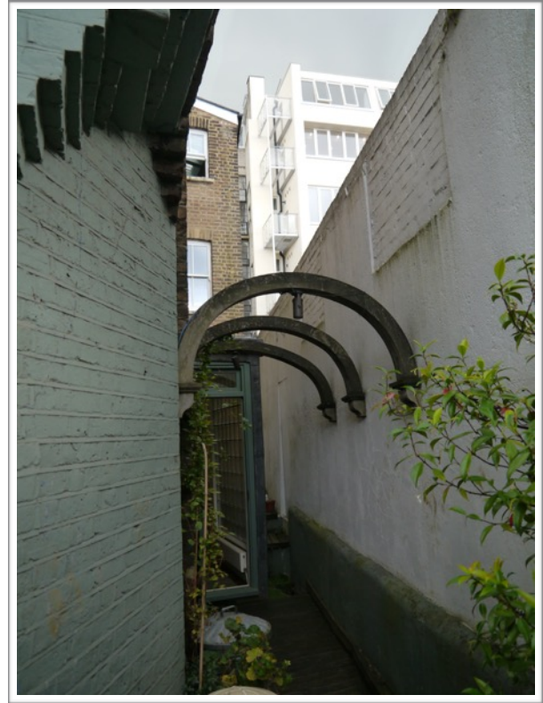
High wall to the right with the rear of 25-26 Hampstead High Street beyond with the new balconies under construction.
