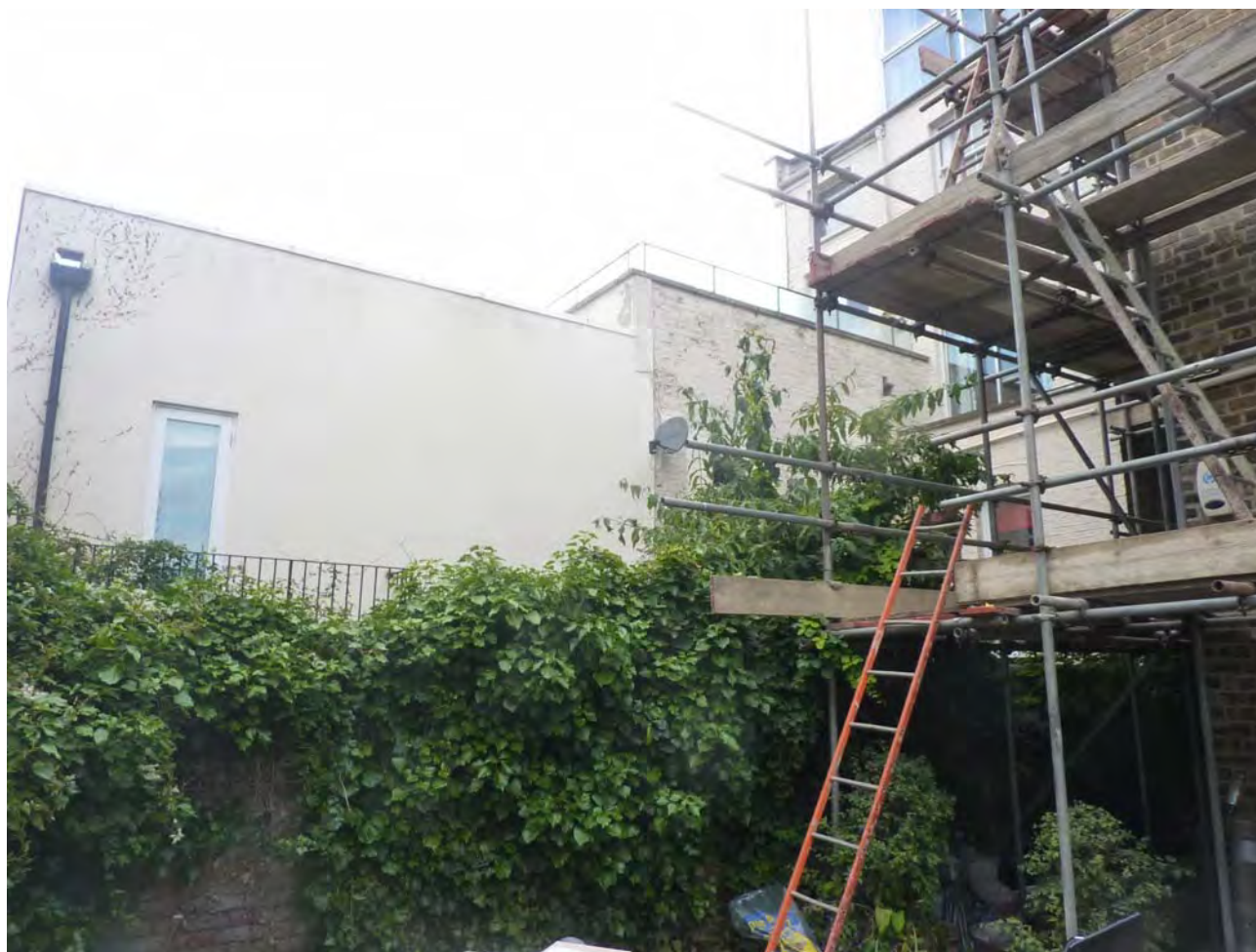
Existing view from rear of 34 Bisham Gardens towards neighbouring 36 Bisham Gardens existing large rear extensions.
