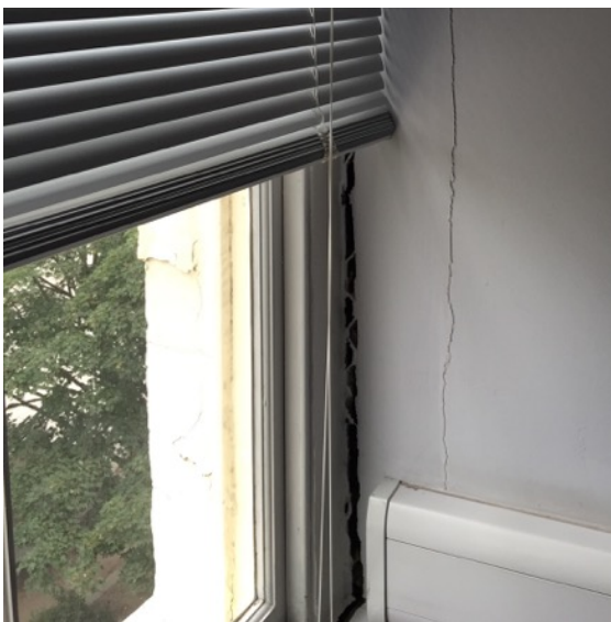
Crack Between Front Facade and Partition at Third Floor
