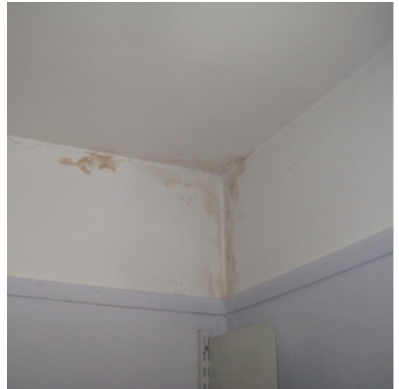
Water Ingress at Corner of Rear/Flank Walls
