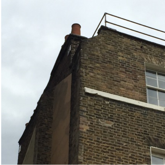
Front Facade Previous Repair Works
