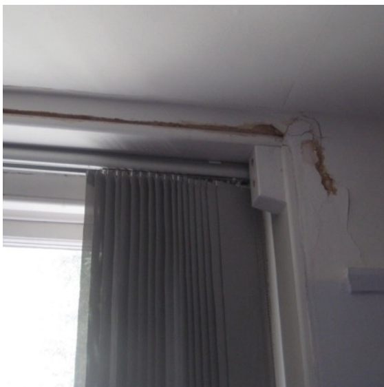
Water Ingress at Head of Window
