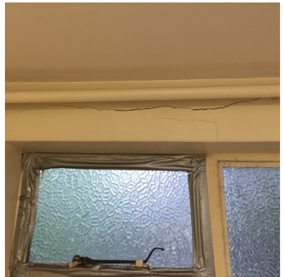
Crack above rear extension window
