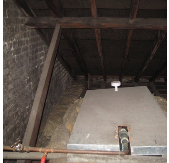
Loft Water Tanks
