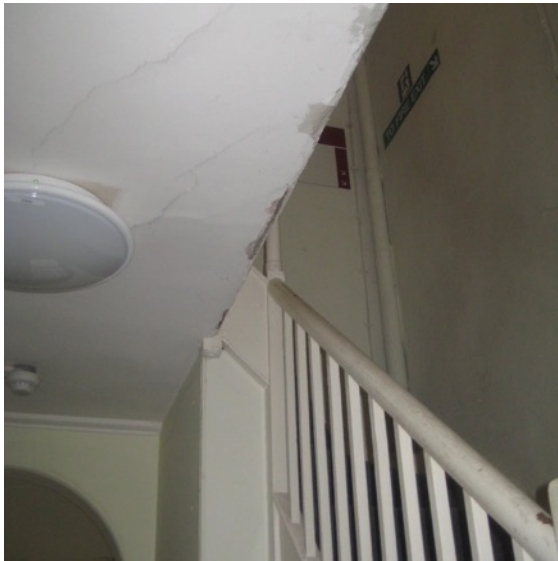
Cracks in Ceiling
