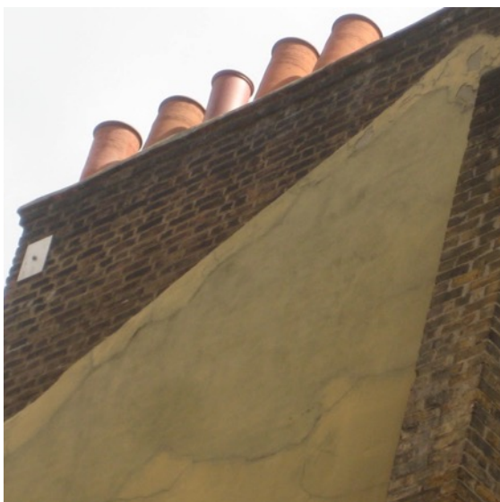
Cracks in Flank Wall Render
