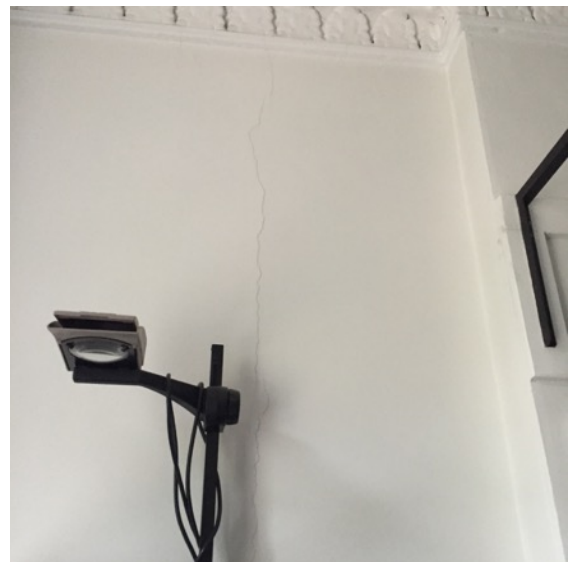
Crack in First Floor Flank Wall
