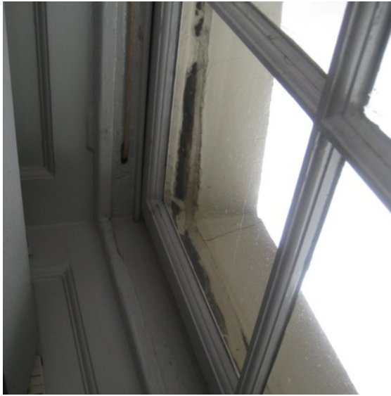
Delamination of Front Facade
