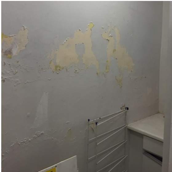
Dampness on rear extension wall
