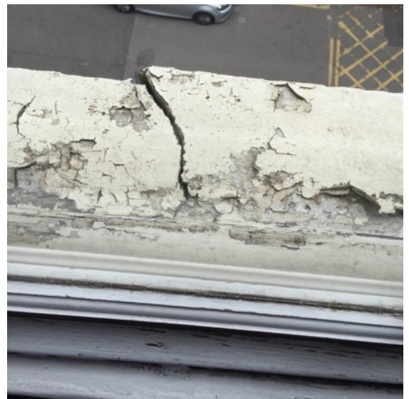
Crack Through Third Floor Window Cill
