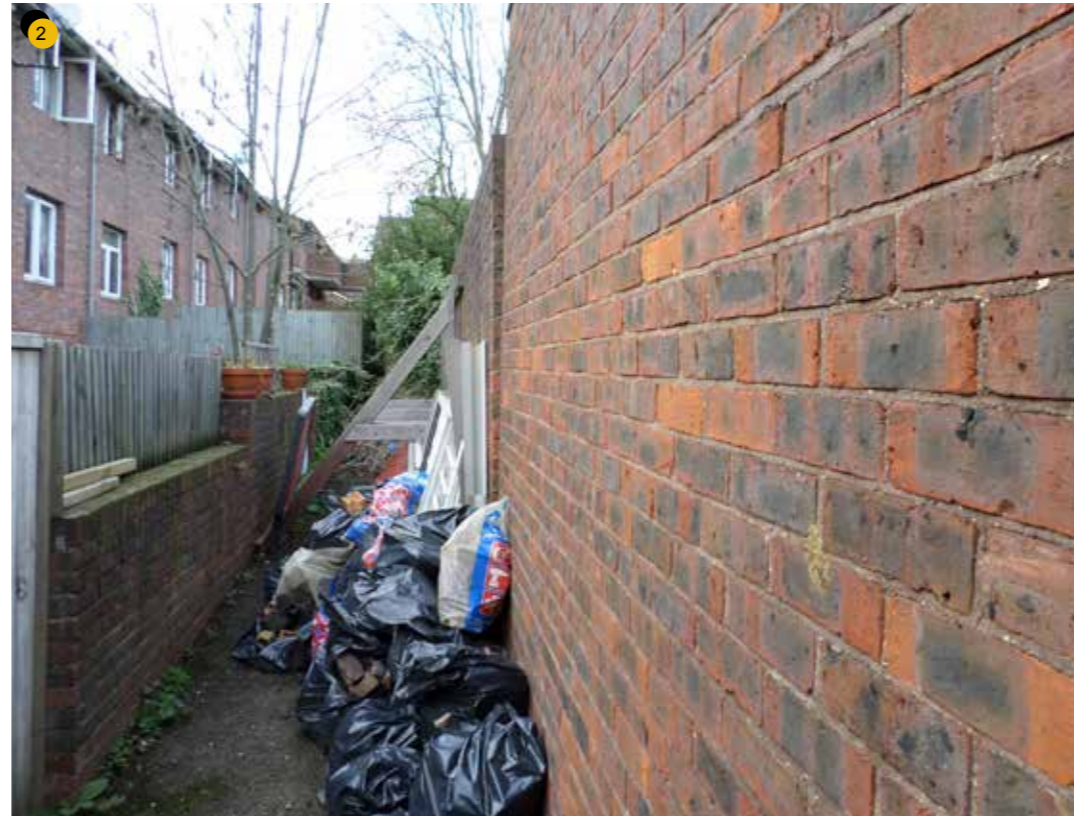
Gated private alleyway down the western edge of the site currently full of building waste and showing signs of collapse
