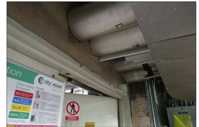
6—Existing plant above rear doors into next room
