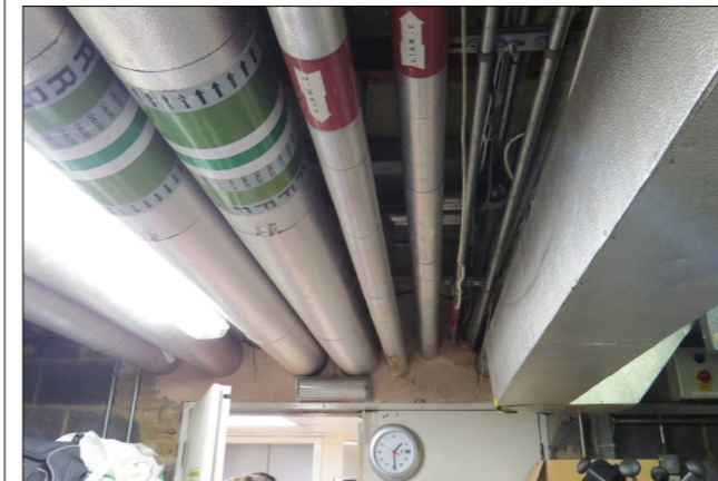
5—Existing plant above main doors into room
