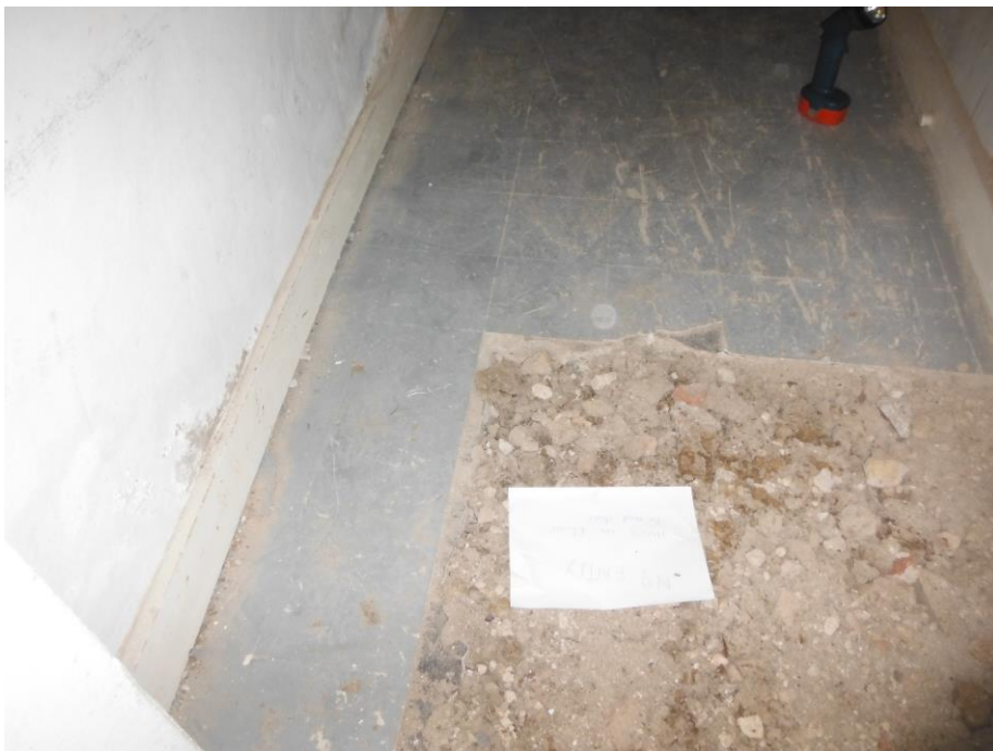
Photo 10 Ground floor lobby adjacent electrical switch room Asbestos floor tiles (assume throughout)
