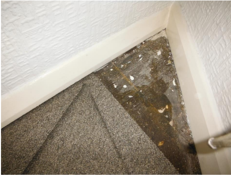
Photo 29 2 nd floor Room 205 Far triangular room Asbestos floor tiles below carpet (assumed throughout)
