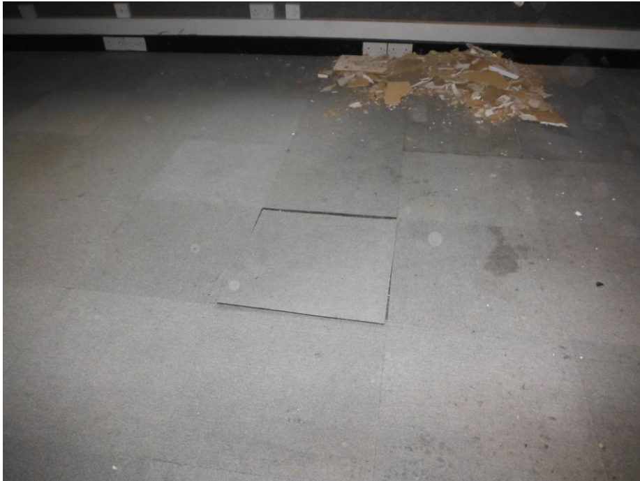
Photo 21 1 st floor Room 107 – Asbestos floor tiles below carpet (assume throughout)
