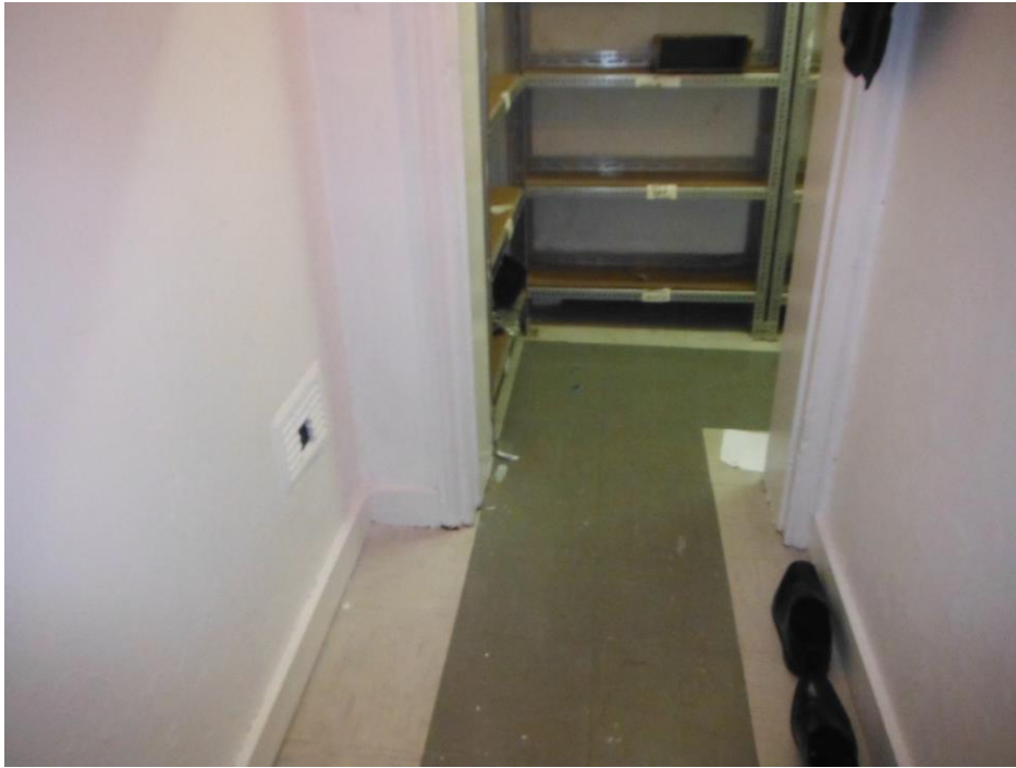
Photo 17 Ground floor room 16 – RHS store room – Asbestos floor tiles
