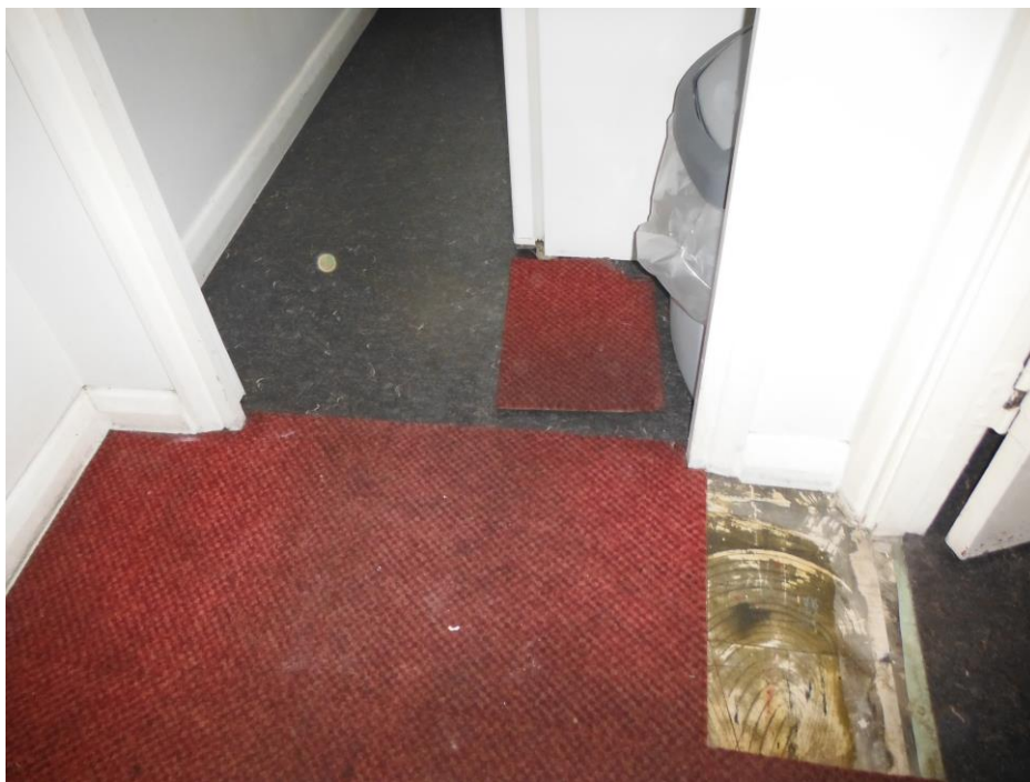
Photo 20 1 st floor lobby adjacent kitchen Asbestos floor tiles below carpet (assume throughout)
