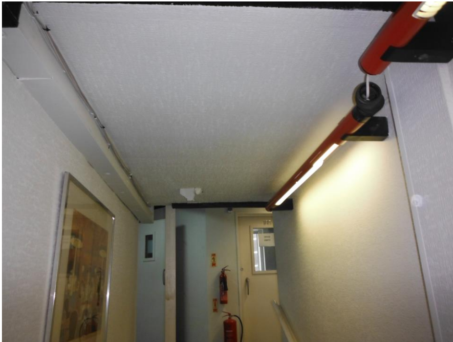
Photo 27 1 st floor landing to fire escape - Asbestos insulating board ceiling panels
