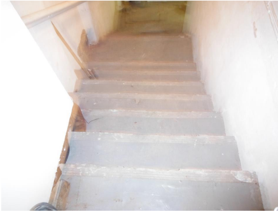
Photo 11 Stairwell to basement - Asbestos floor tiles (assume throughout)
