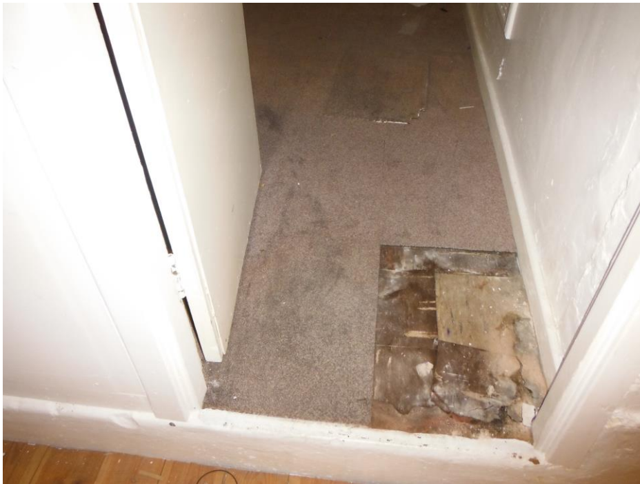
Photo 18 Ground floor room 16 – LHS store room – Asbestos floor tiles below carpet
