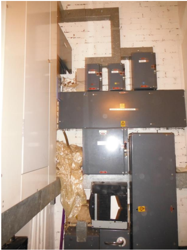
Photo 5 Ground floor Electrical switch room (plant not accessed) Asbestos tape pads to fuses (assumed)
