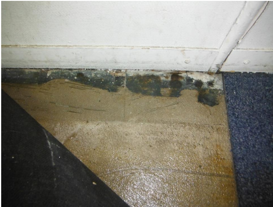
Photo 7 Ground floor reception room - Asbestos floor tiles (assume throughout)
