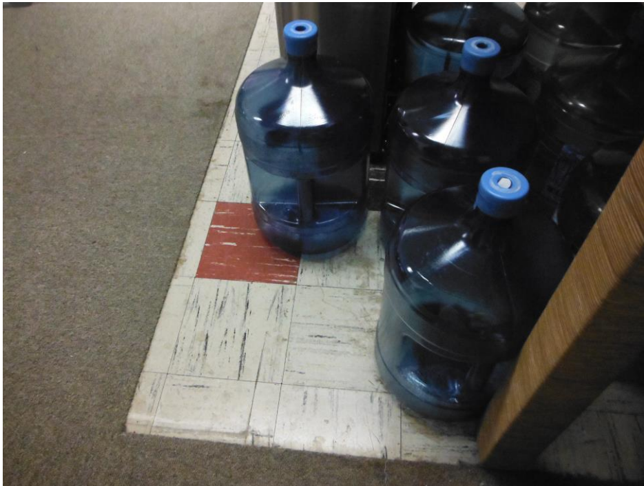
Photo 31 2 nd floor Open plan office room 201 – Asbestos floor tiles (assumed throughout)
