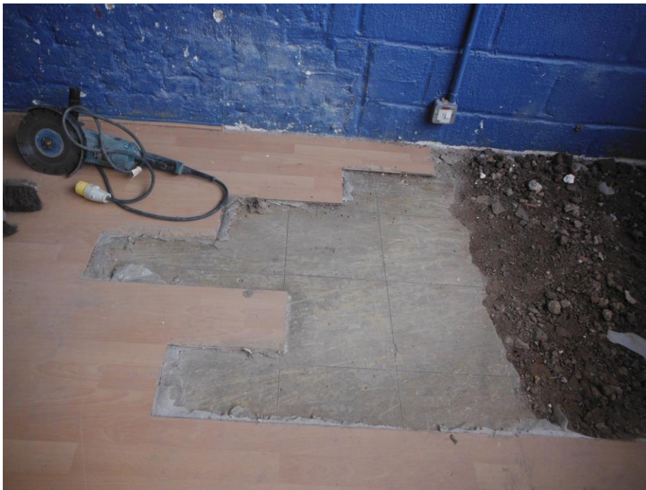
Photo 4 Ground floor – 2 nd workshop room – Asbestos floor tiles (assumed throughout)
