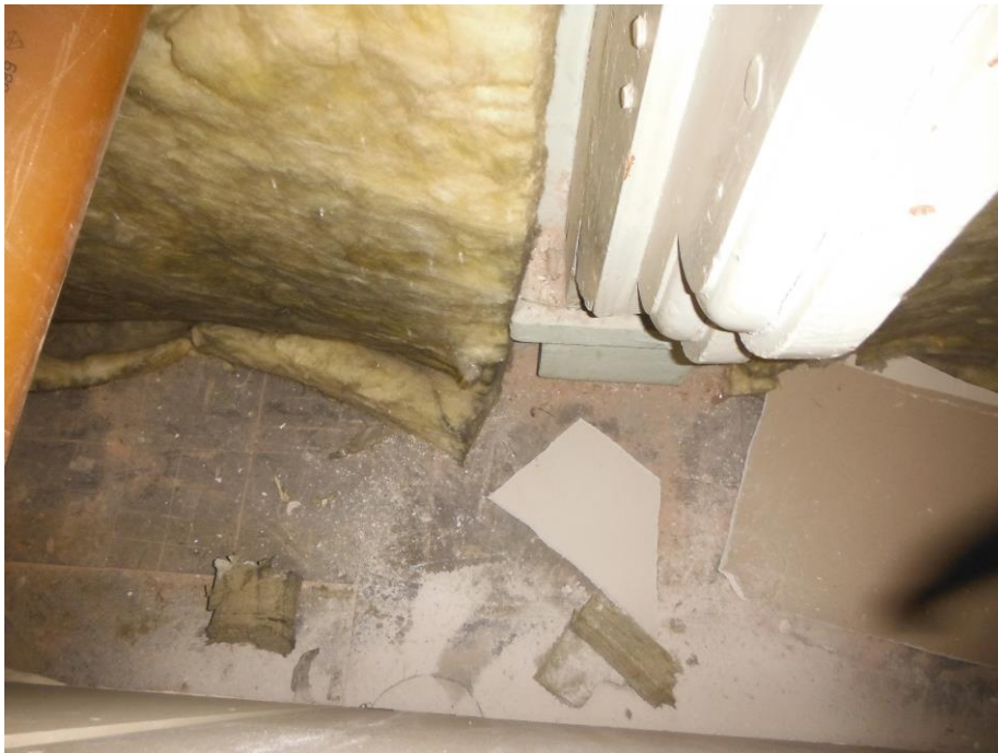
Photo 30 2 nd floor Room 202 Asbestos floor tiles within voids in sides of room (assume throughout)
