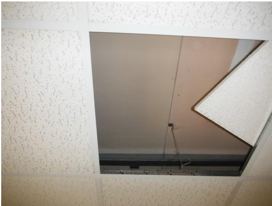
Photo 28 1 st floor Room 116 - Asbestos bevelled edged fibreboard ceiling tiles above suspended ceiling (assumed throughout)
