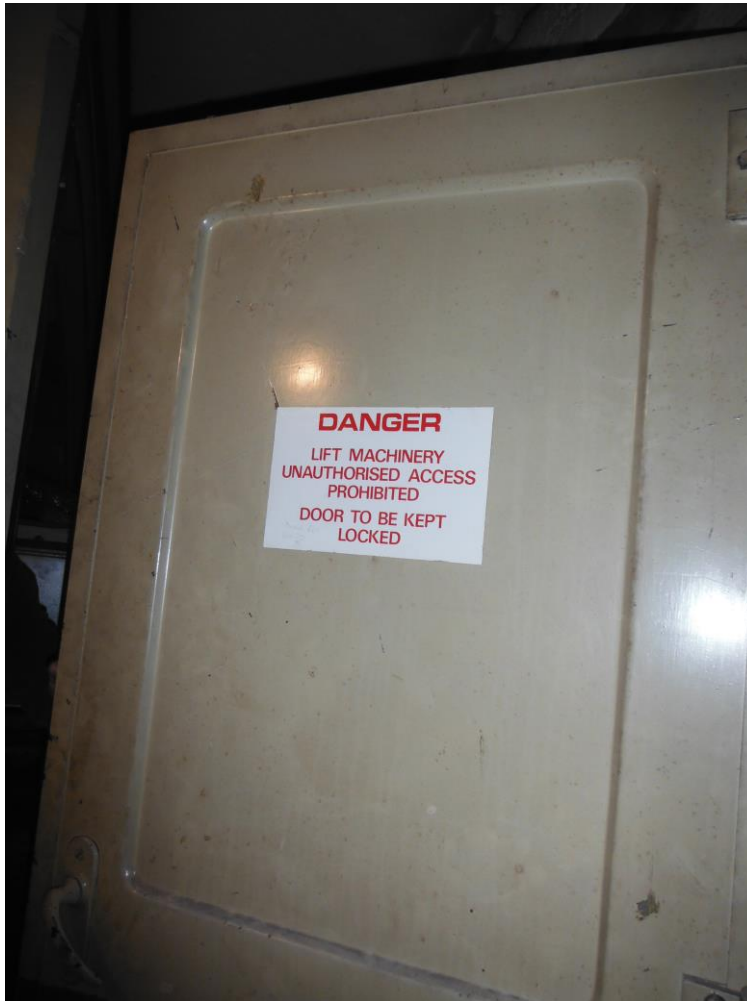
Photo 33 Roof space Lift motor room – Asbestos fire door (assumed)
