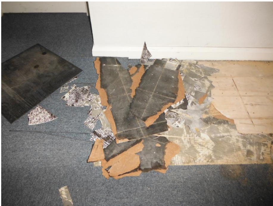
Photo 22 1 st floor Lobby adjacent room 105 – Asbestos floor tiles debris
