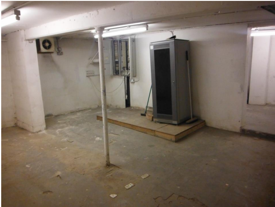
Photo 13 Basement - Asbestos floor tiles (assume throughout)
