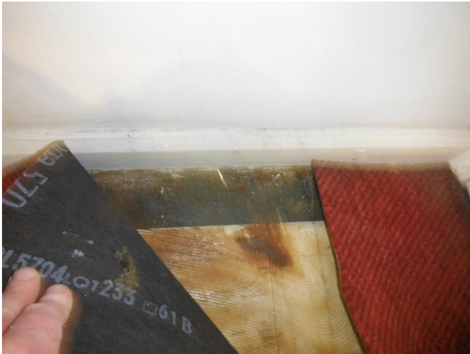
Photo 9 Ground floor waiting area - Asbestos floor tiles (assume throughout)
