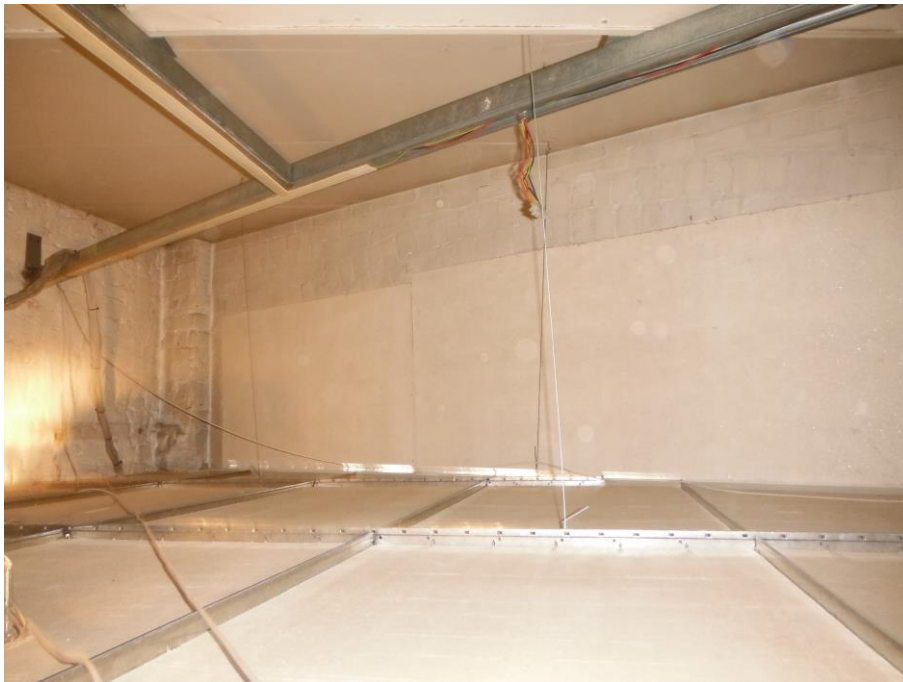
Photo 6 Ground floor 2 nd workshop room Non asbestos supalux panels above windows in ceiling void
