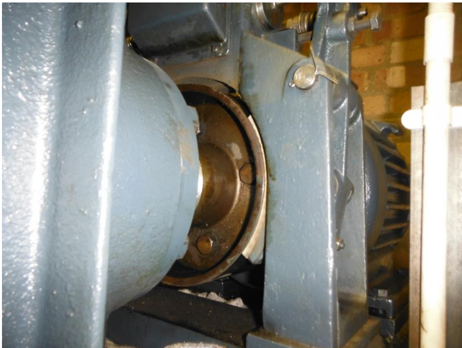
Photo 32 Roof space Lift motor room – Asbestos cement brake shoe linings (assumed)
