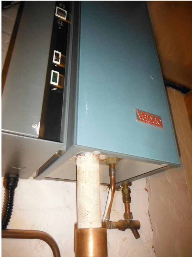
Photo 19 Room 16 Switch cupboard – Non asbestos rope lining to Vapac unit
