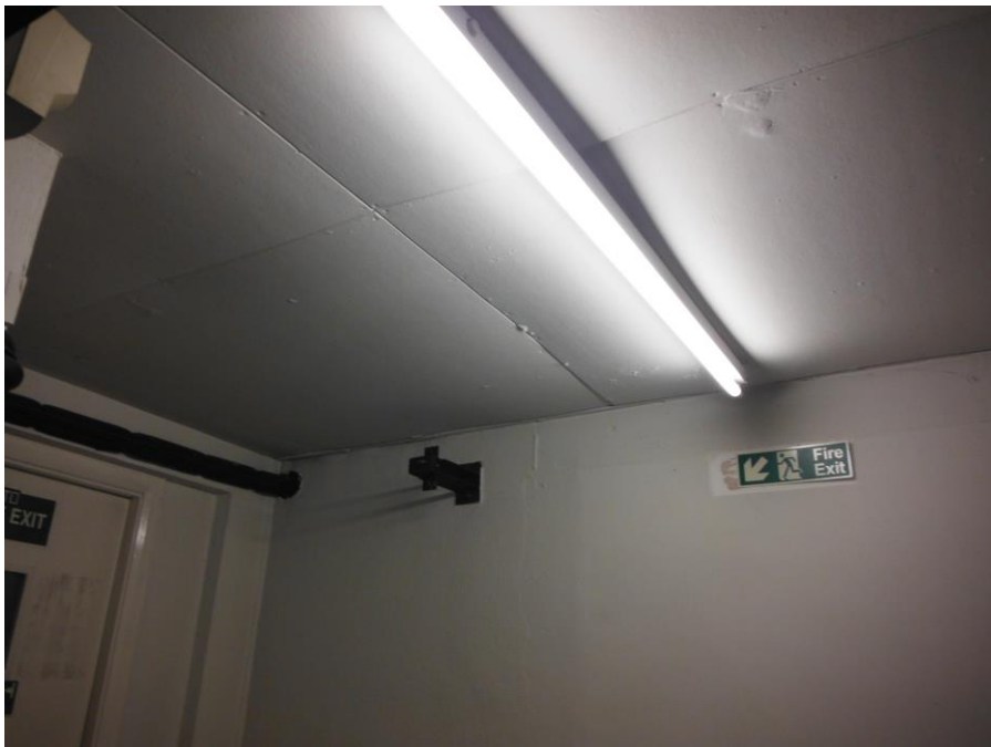
Photo 26 1 st floor landing to fire escape Asbestos bevelled edged fibreboard ceiling tiles (assumed throughout)
