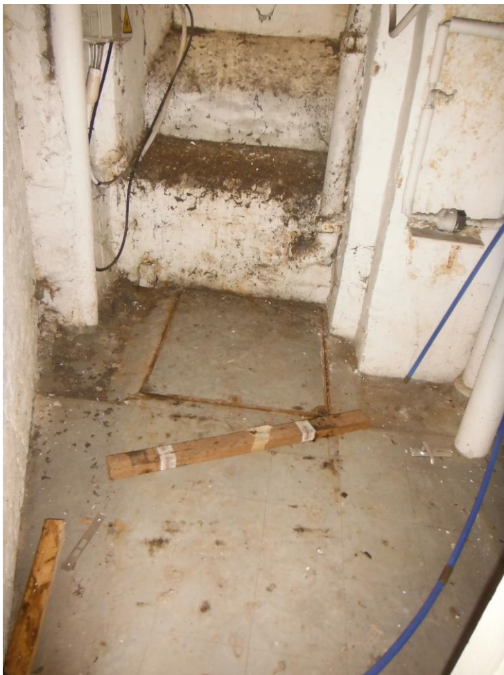
Photo 14 Basement - Asbestos floor tiles (assume throughout)
