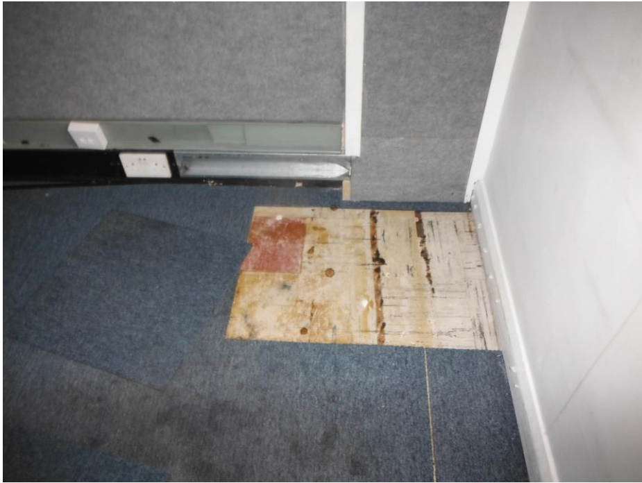
Photo 23 1 st floor Room 104 – Asbestos floor tiles below carpet (assume throughout)
