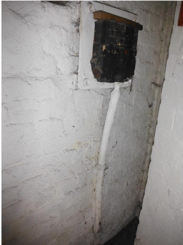
Photo 1 Ground floor loading bay – Non asbestos bitumen rope lining to mains electrical cable
