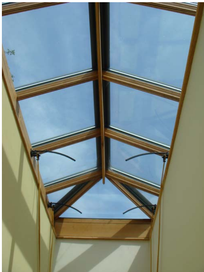
Glazed roof lantern built smaller than approved (length reduced)
