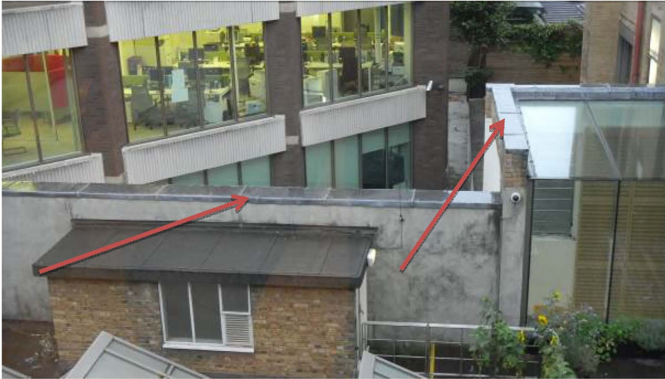
This photo of the rear of the property showing a similar treatment adopted to the caps of parapet walls.
