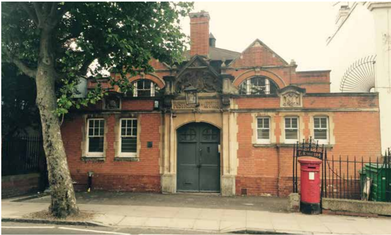
Fig. 13 Front facade as existing showing general state of disrepair.
