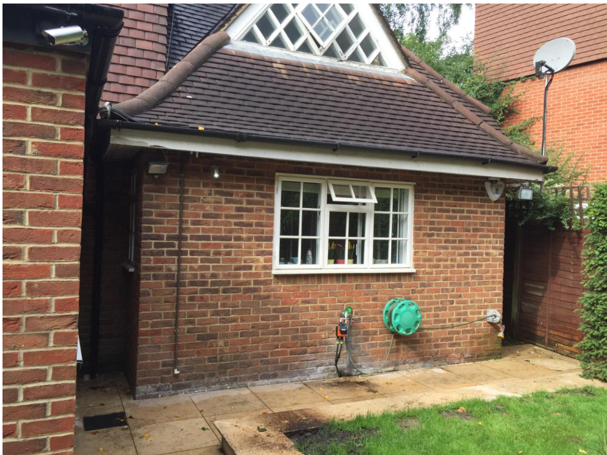
Image showing existing rear window (kitchen window) to be replaced with a french patio door
