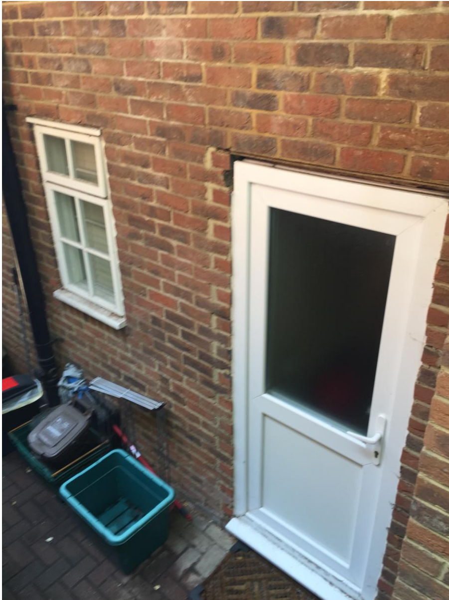
Image showing existing side (north) elevation - side door to be removed and opening to be blocked up using matching bricks
