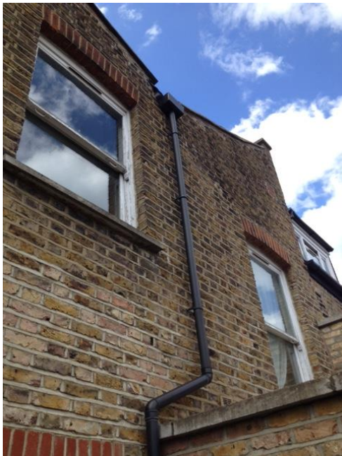
2- View from existing terrace towards roof and proposed site of rear extension
