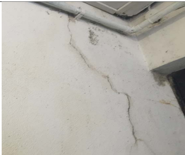
Figure 9: Cracking on garage walls
