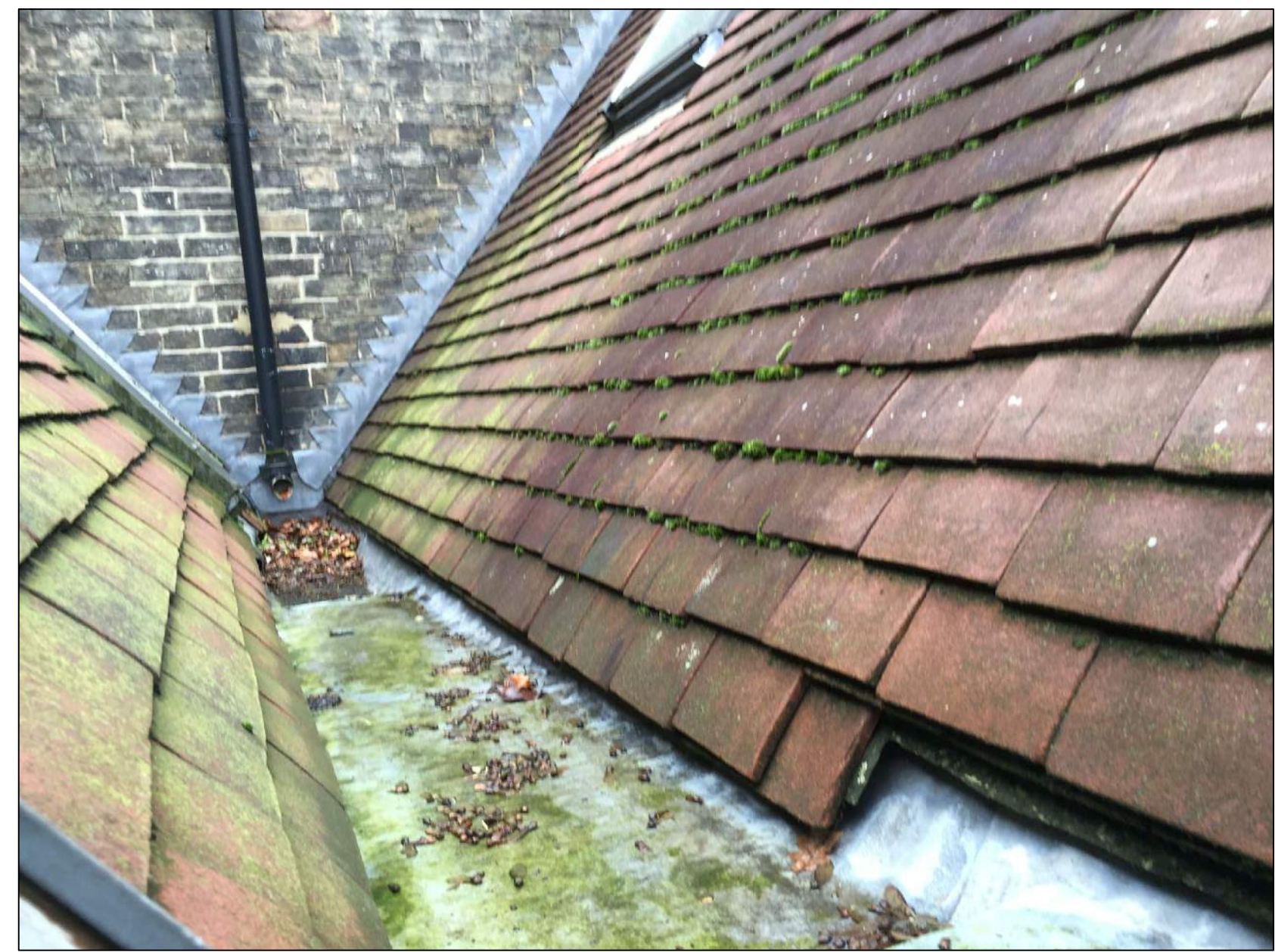
PHOTO B PROPOSED LOCATION FOR NEW EXTERNAL CONDENSER
