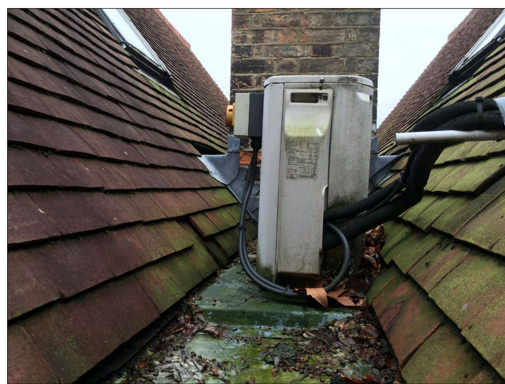
PHOTO A EXISTING ROOF MOUNTED EXTERNAL CONDENSER
