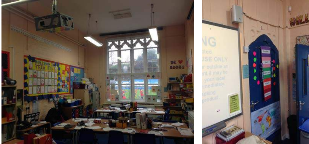
Year 6 Classroom. The room was enlarged in 1888 and the window reinstated without its original diamond panes of glass.
