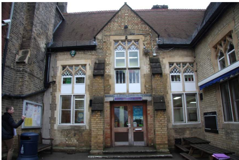
South elevation of school showing main entrance doors, inserted in place of the original windows in the 1970s
