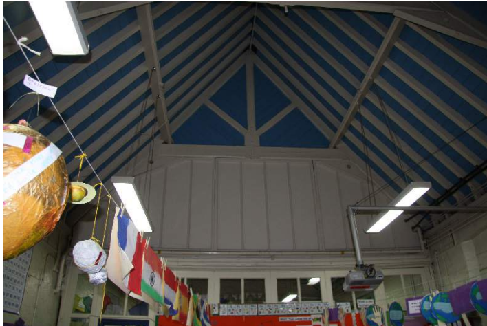
The roof and screen in the Year 2 Classroom, originally the infant schoolroom
