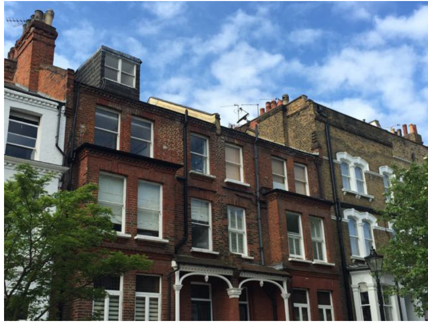
21 Carlingford Road, NW3. The existing dormer is narrow & in poor repair.
