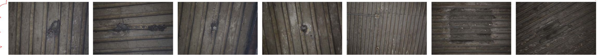
Photos 1-3 SE Condition Survey Reference 7 'Numerous areas of spalled concrete and previous repairs' Photo 4 SE Condition Survey Reference 8 'Hole through soffit' Photo 5 SE Condition Survey Reference 12 'Remnants of past fixings. Rust staining present.' Photo 6 SE Condition Survey Reference 23 'Patch repair exposing aggregates' (probable infill of hole in slab, see key) Photo 7 SE Condition Survey Reference 8 'Previous repair. Potential risk of spalling'
